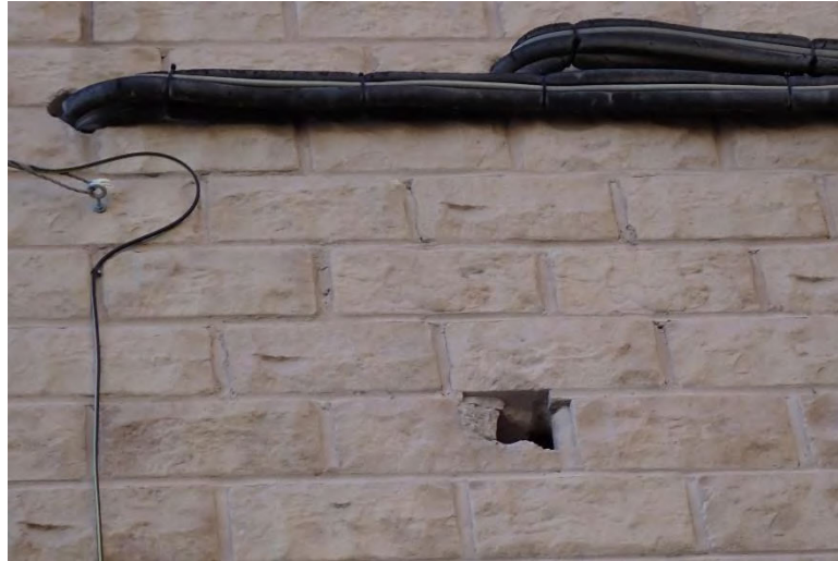
A hole in the block-work wall ( Target Note 12 ).
