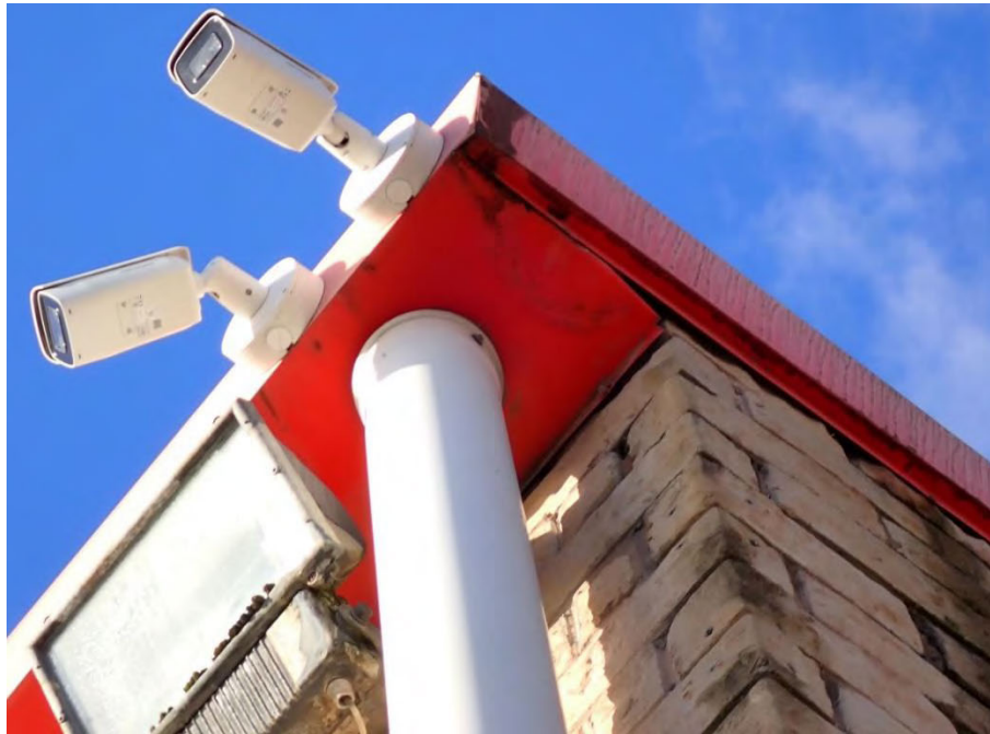
A gap at the wall top ( Target Note 12 ). Note the flood-light.
