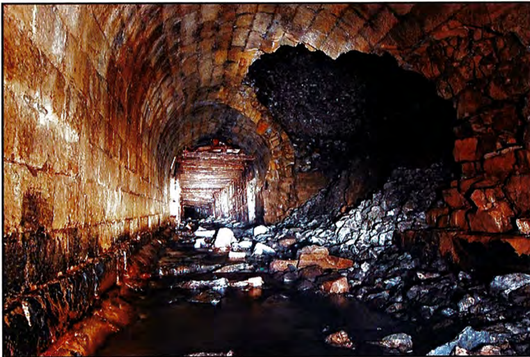
Well-constructed roadway with collapse
