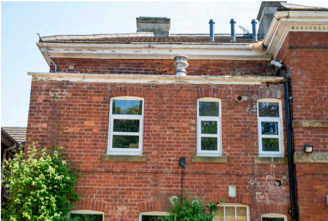
Photograph 9: The brickwork is punctured by holes and some of the bricks have been shattered by frost. However, no bats were seen to enter or leave this part of the building.
