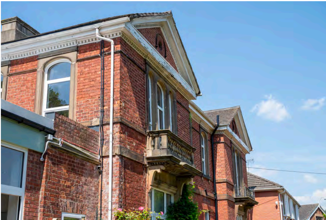
Photograph 7: Much of the entablature is rotting.
