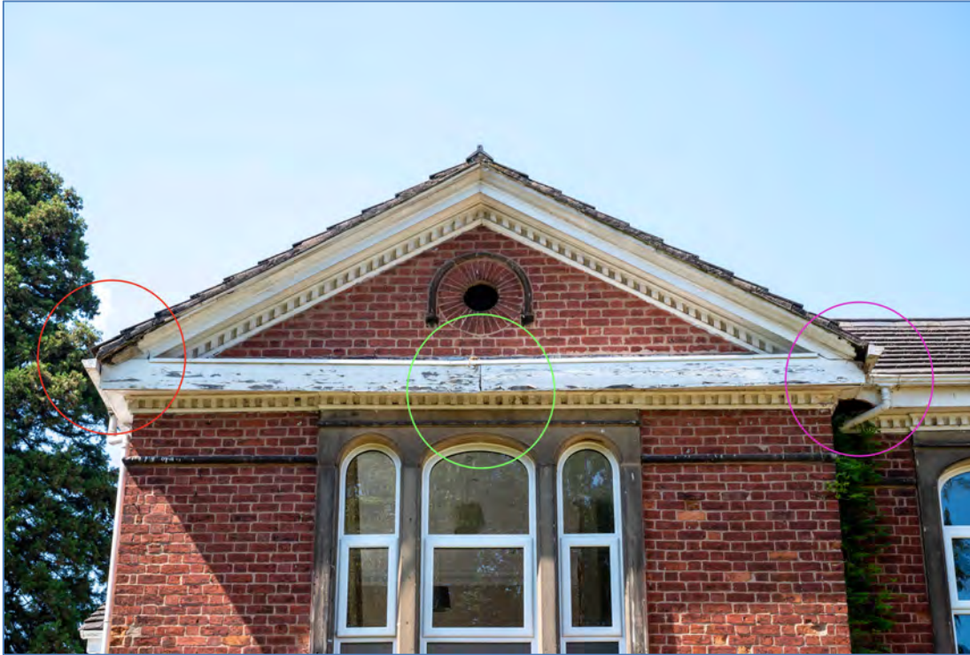
Photograph 15: We have seen bats emerge and enter the cavity circled in red. Bats may also be entering the cavity circled in purple.
