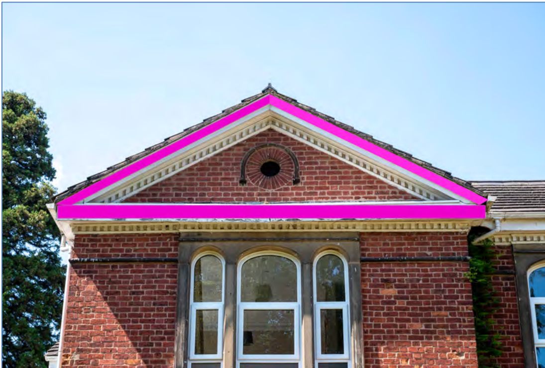
Photograph 16: We anticipate that the areas highlighted in magenta will need to be replaced with new timber.
