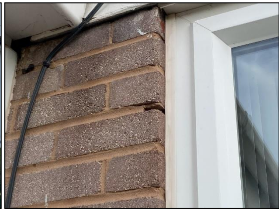
Photograph 2 showing a minor gap in the brickwork
