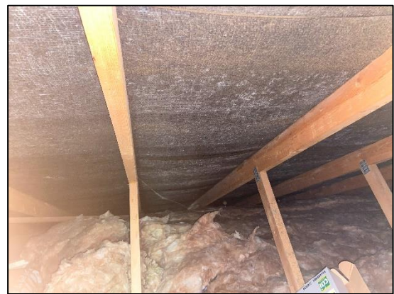
Photograph 10 showing the mould growth on the lining
