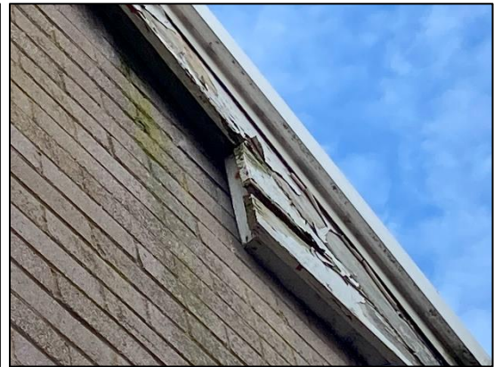
Photograph 6 showing minor areas of water damage
