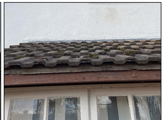
Photograph 4 showing the gaps under the extension tiles
