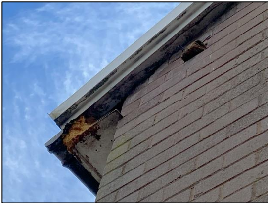
Photograph 5 showing an area of water damage
