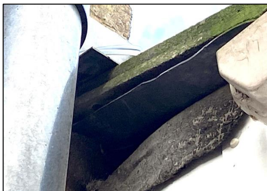
Photograph 7 showing the gap between the extension and the main house
