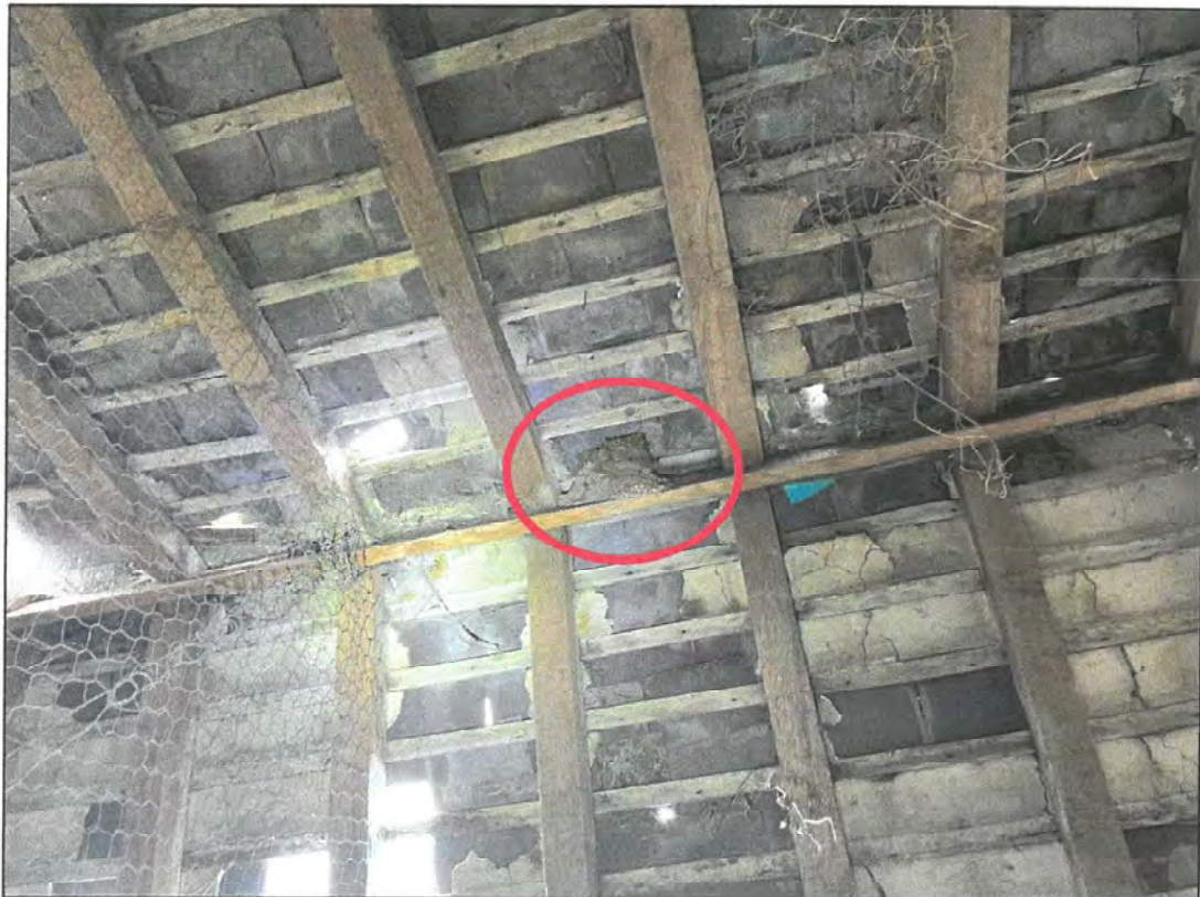
Plate 14 – Swallow nest within the structure
