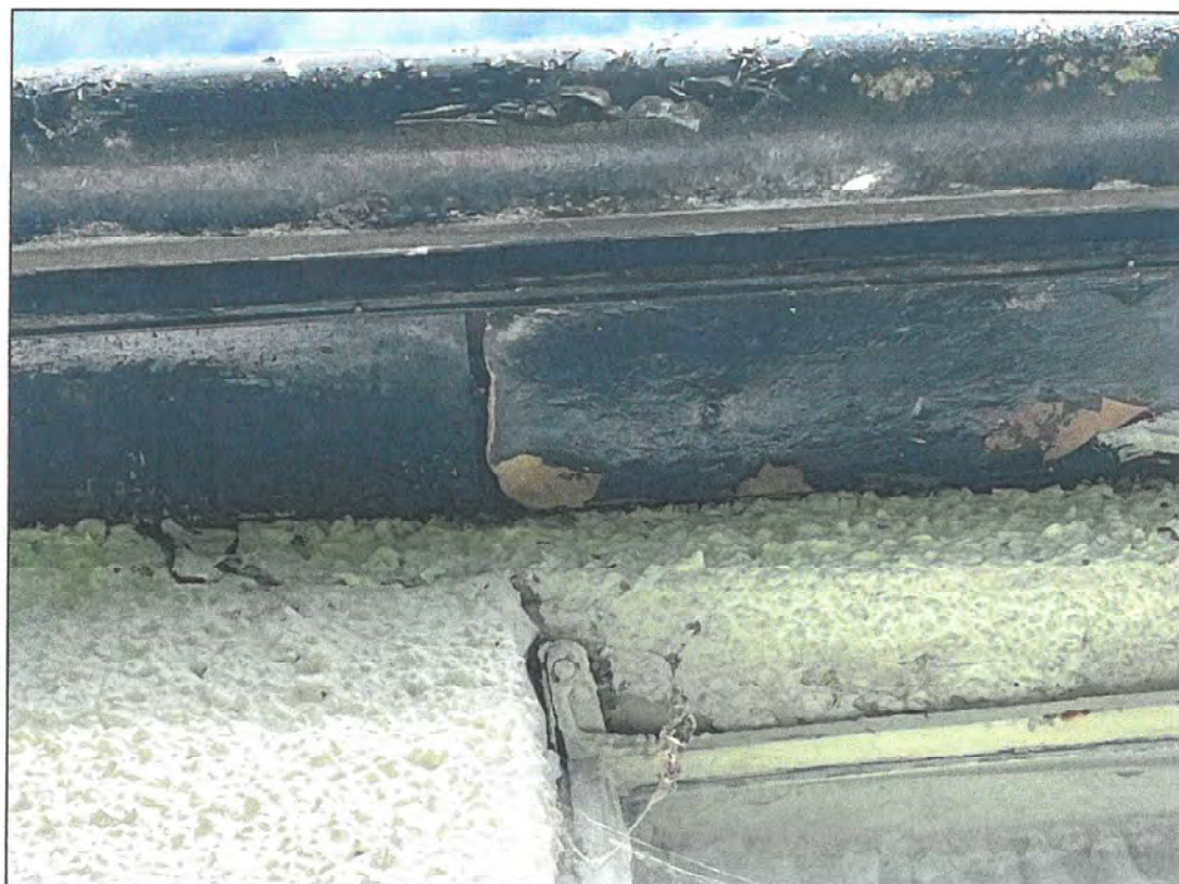
Plate 8 – Gap in soffit on southern elevation
