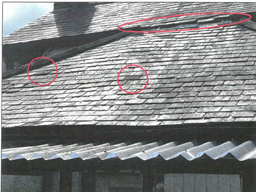
Plate 7 – PRFs where the hipped roof meets the pitched roof, alongside several slipped slates
