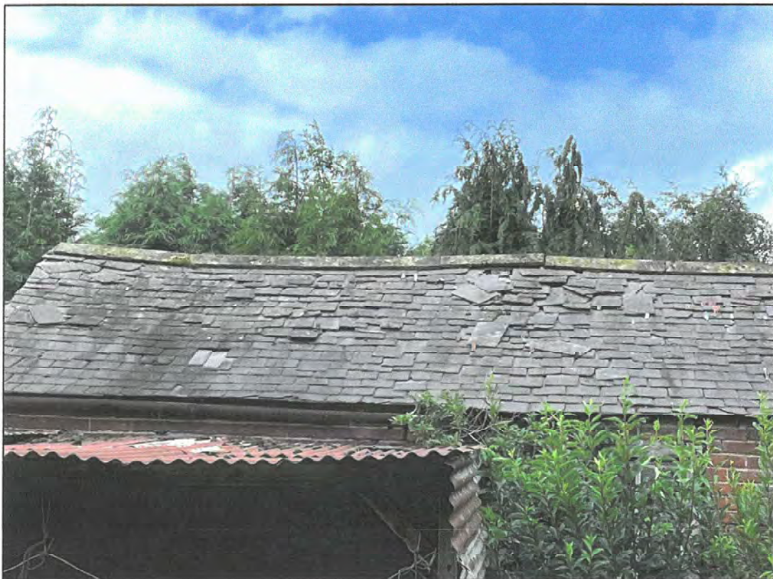
Plate 16 – PRFs in the slates and ridge tiles on the outbuilding
