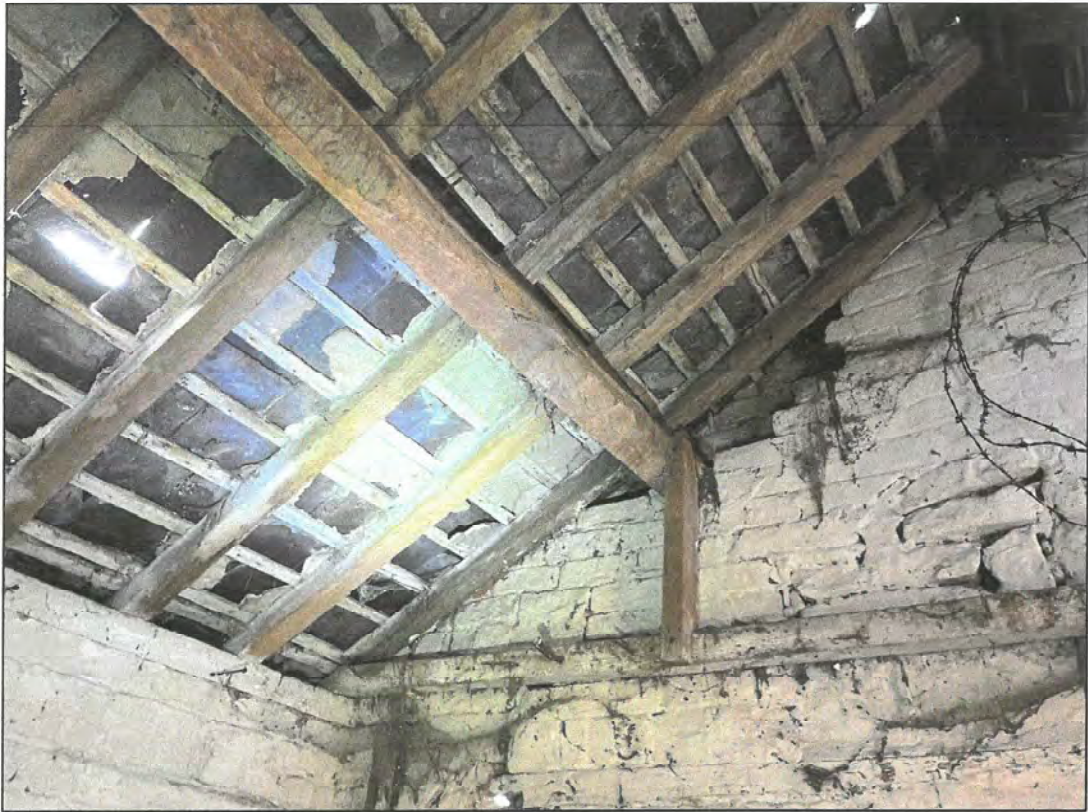
Plate 15 – Degraded mortar in outbuilding and gaps in slates evident
