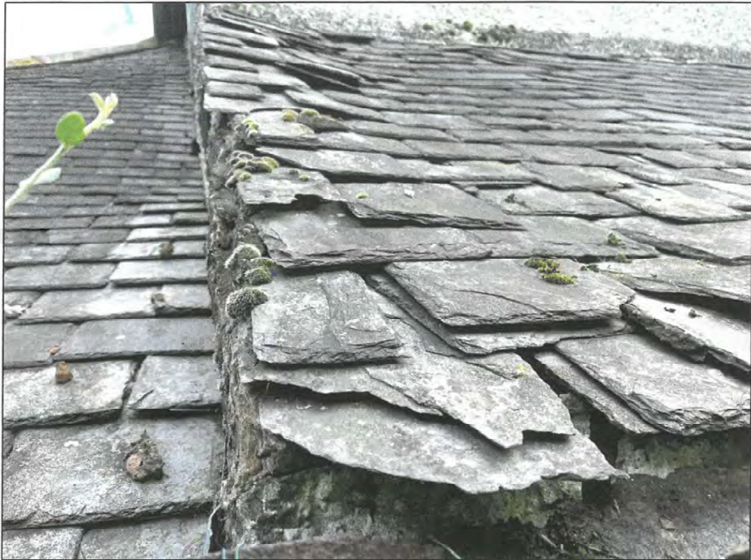
Plate 9 – Numerous lifted slates on western aspect
