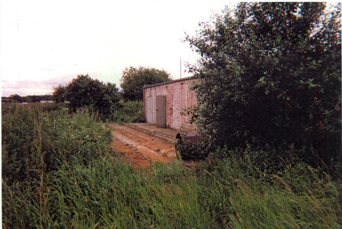
Plate 12 Interceptor pit at the end of the french drain running along the western boundary of the site. Iron staining can be seen around the pit.
