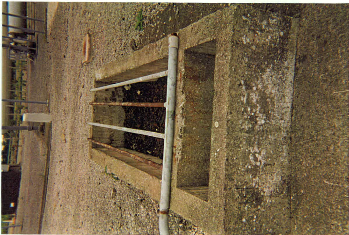
Plate 9. A coke filter located in the area of the former Benzol Plant.
