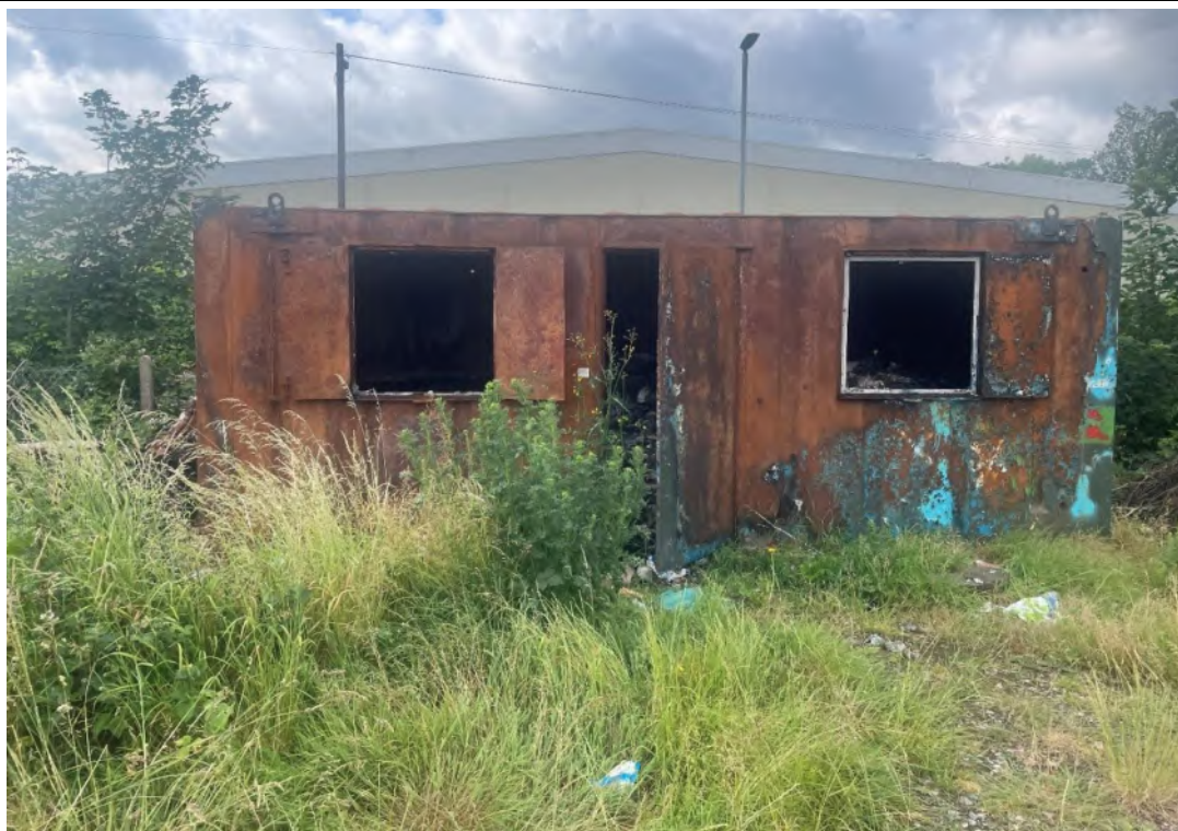
Photo 14 – Old container present along southern boundary. Evidence of fire damage. Burnt ash material present inside container. No evidence of any impact outside the container.
