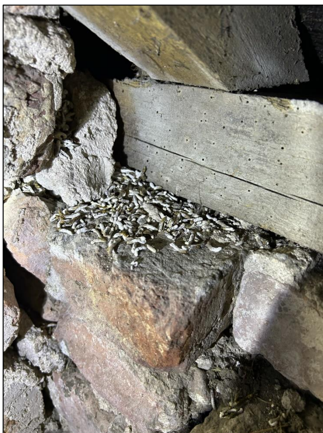
Plate 10 – Bird droppings in the loft, indicative of sparrow usage
