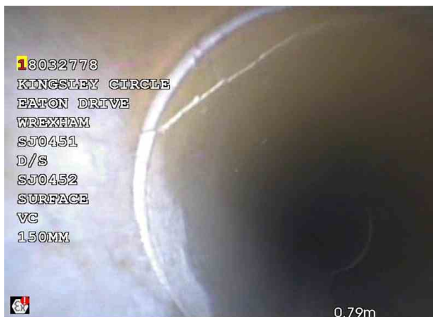
1_SJ0451_SJ0542.jpg, 00:00:04, 0.48 m Fracture, circumferential at joint from 10 o'clock to 2 o'clock
