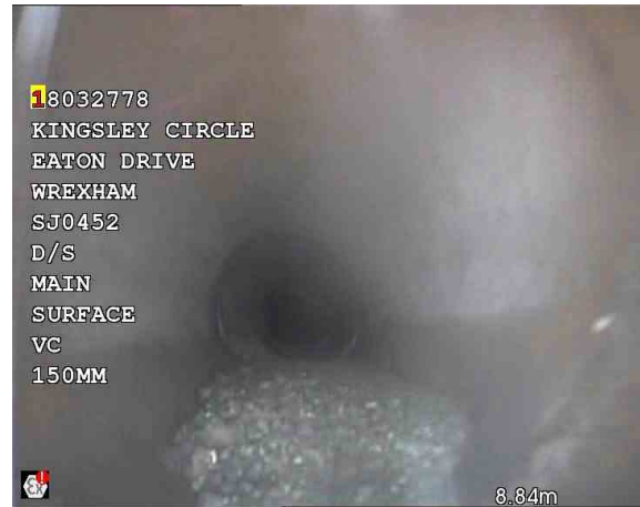
SJ0542X_c10e0930-6a47-449b-b98d-a363c4a99fd1_20240301_091229_308.jpg, 00:00:40, 8.84 m Settled deposits, coarse, 20% cross-sectional area loss
