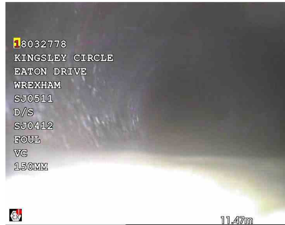
SJ0511X_e4d35471-ab61-42d3-a042-d57c73febdfe_20240301_092846_152.jpg, 00:00:27, 11.47 m Attached deposits, fouling from 5 o'clock to 7 o'clock, 10% cross-sectional area loss, start
