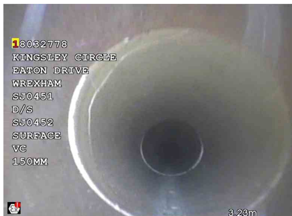
SJ0451X_5130bcdb-e9bb-4227-9cec-b6ff4069ea8d_20240229_135838_219.jpg, 00:00:10, 3.23 m Fracture, circumferential at joint from 8 o'clock to 1 o'clock
