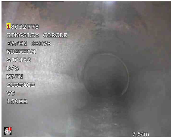
SJ0542X_87ebbb8c-8673-4f92-aaf4-1be037cf3409_20240301_091208_562.jpg, 00:00:25, 7.44 m Settled deposits, fine, 5% cross-sectional area loss, start
