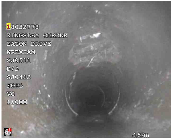
SJ0511X_bc672735-70ef-4b88-bc77-8b9e5d36a7b8_20240301_092819_353.jpg, 00:00:12, 4.57 m Hole in drain or sewer at 12 o'clock, POSSIBLE HOLE
