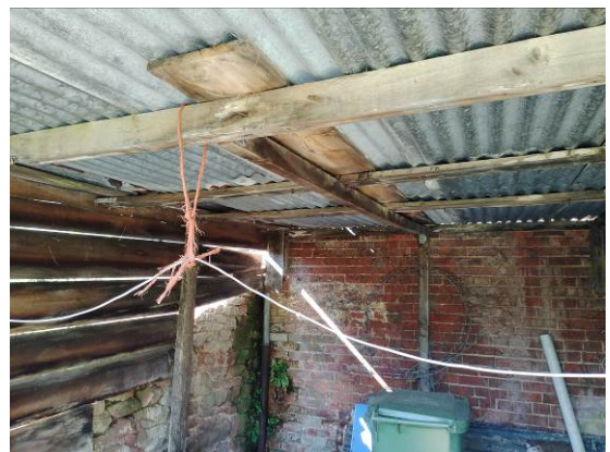
Photo 6 – Staining to elevation due to water cascading downface from roof.
