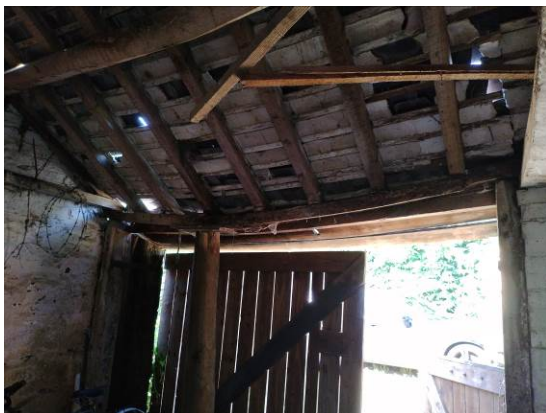
Photo 9 – Severe distortion to door lintel.
