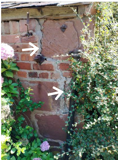
Photo 2 – Cracking at junction with side elevation.
