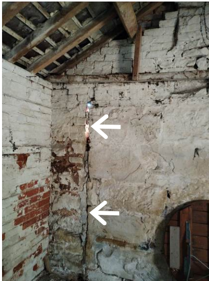
Photo 8 – Gap between masonry and brickwork.
