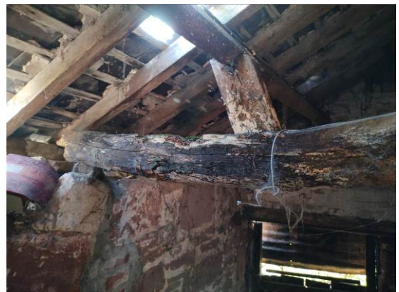
Photo 12 – Severe section losses to beam.
