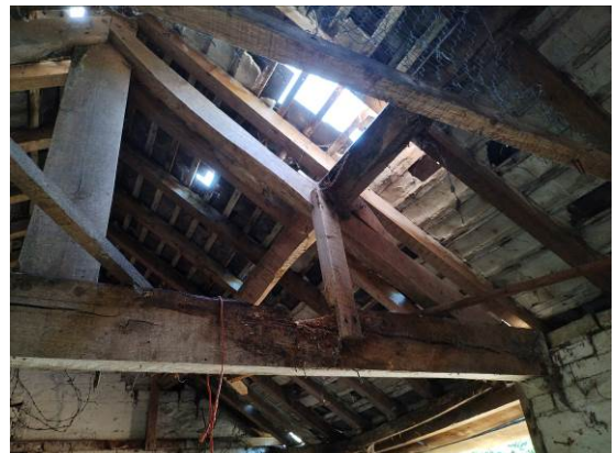
Photo 11 – Staining and section losses to truss.
