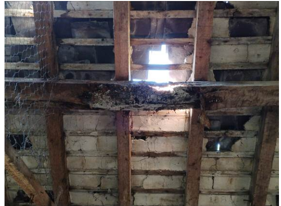
Photo 10 – Staining and section losses to purlin.
