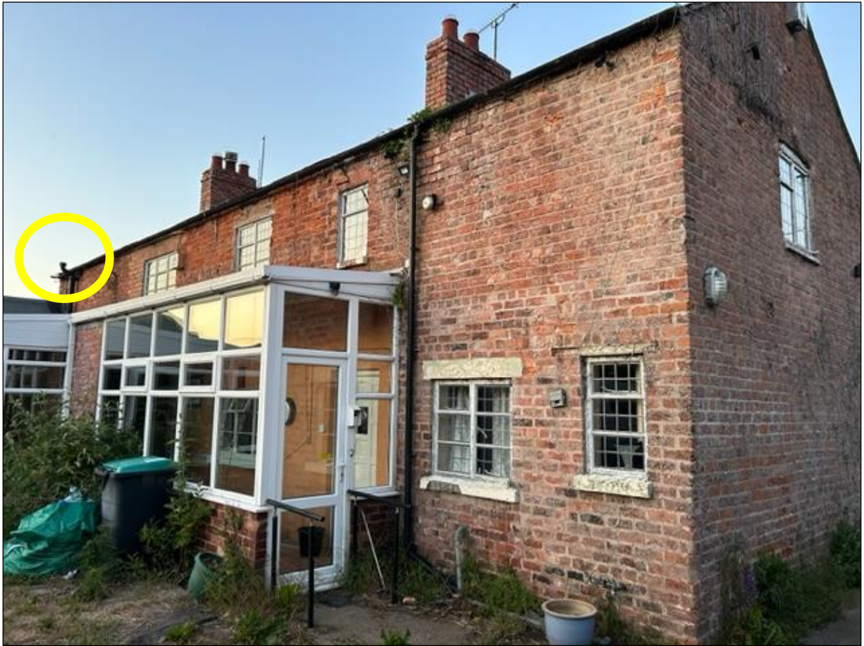
Photograph 1; (Circled) Indicates emergence point.
