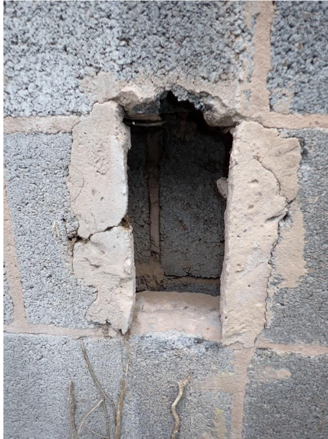
A hole in the block-work on the southwest elevation ( Target Note 10 ).
