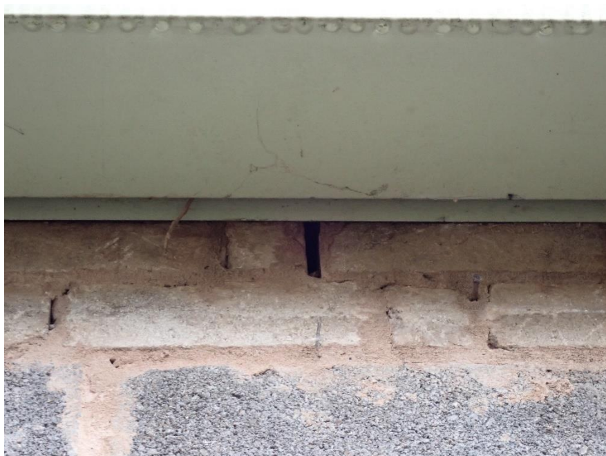
A possible gap at the wall top on the southwest elevation ( Target Note 10 ).
