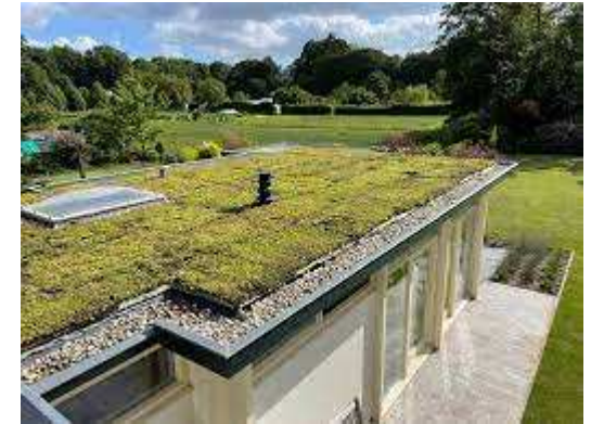
Example of Sedum living roof
