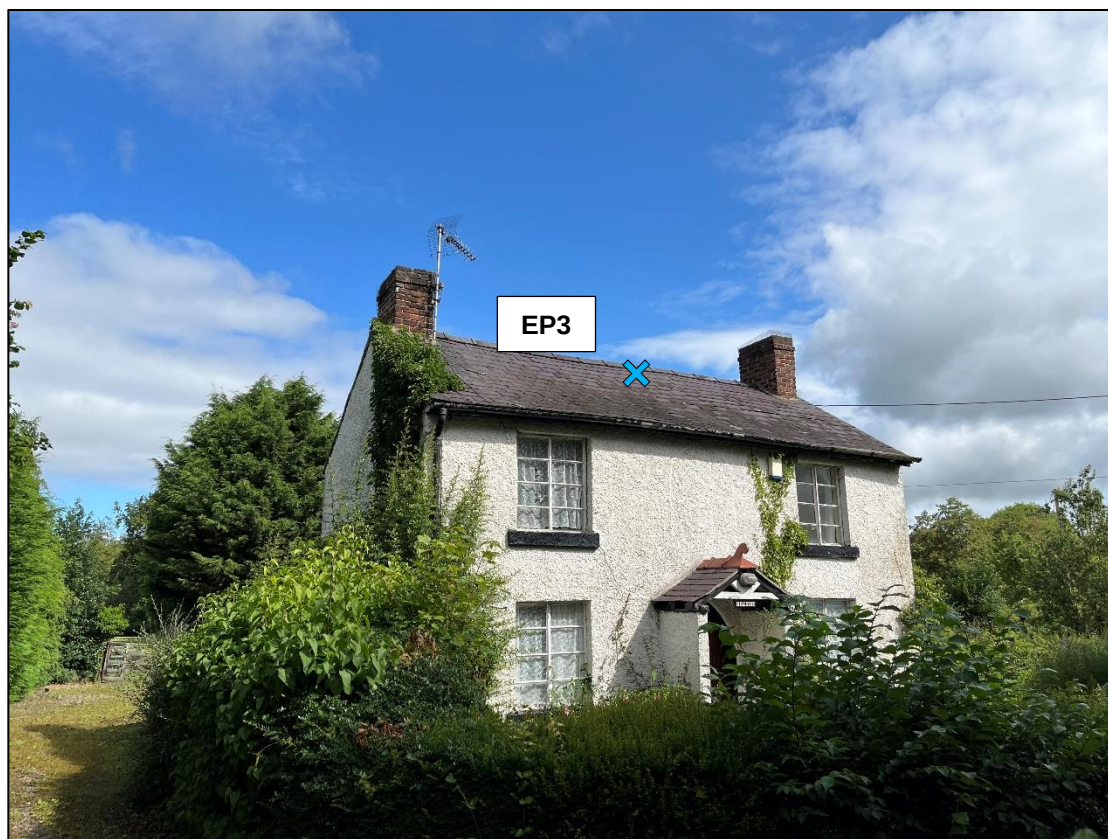
Figure 5.4 – Emergence points 3 from beneath lifted ridge tiles
