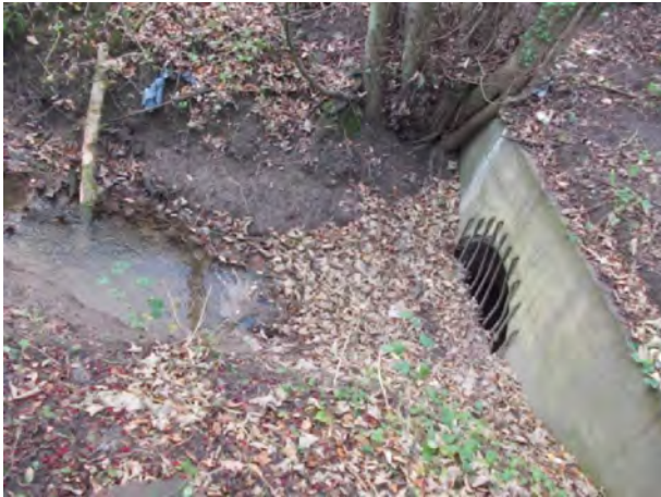
Plate 19: Blocked Culvert in eastern area of Bedwell Brook at site boundary by entrance to site (12-12-2013)
