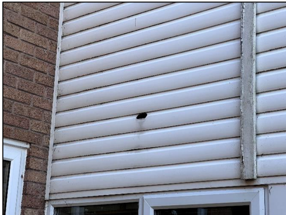
Figure 8: The holes in the uPVC cladding.
