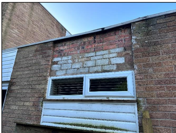
Figure 6: Missing uPVC cladding to the rear of the garage.
