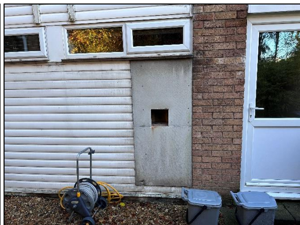
Figure 7: Holes adjacent to the rear door.
