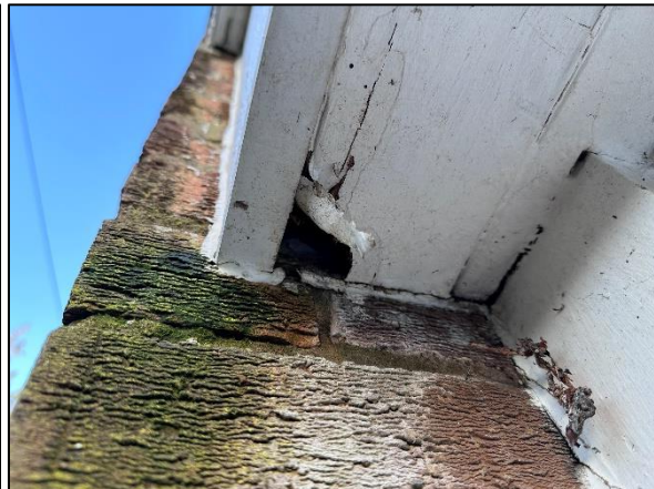
Figure 9: The hole in the soffit over the garage door.
