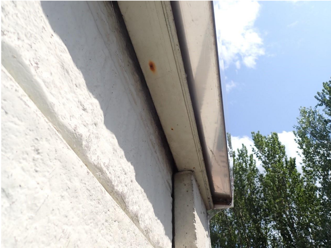
Photograph 11. Gap between the timber soffit and concrete façade on Building 2.
