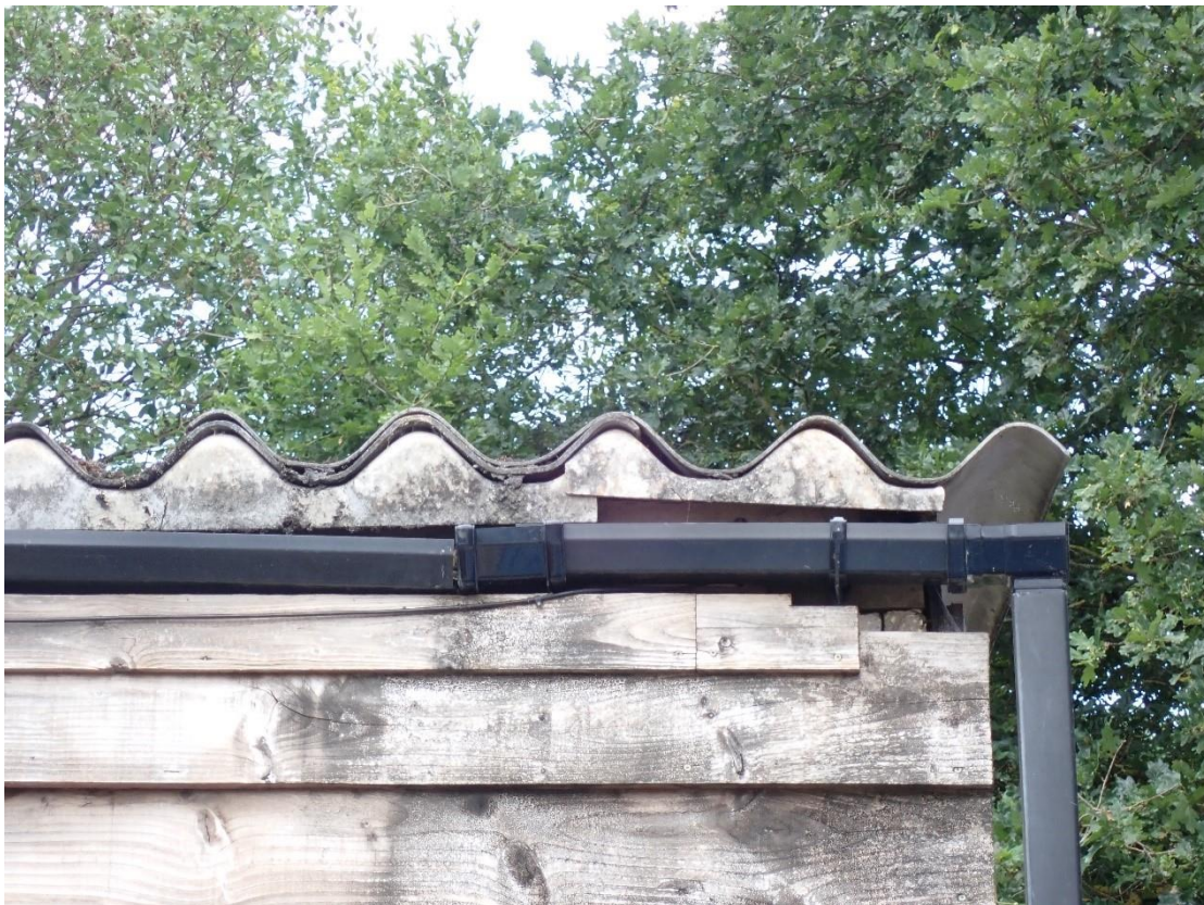
Photograph 8. Lifted asbestos roof on Building 1.
