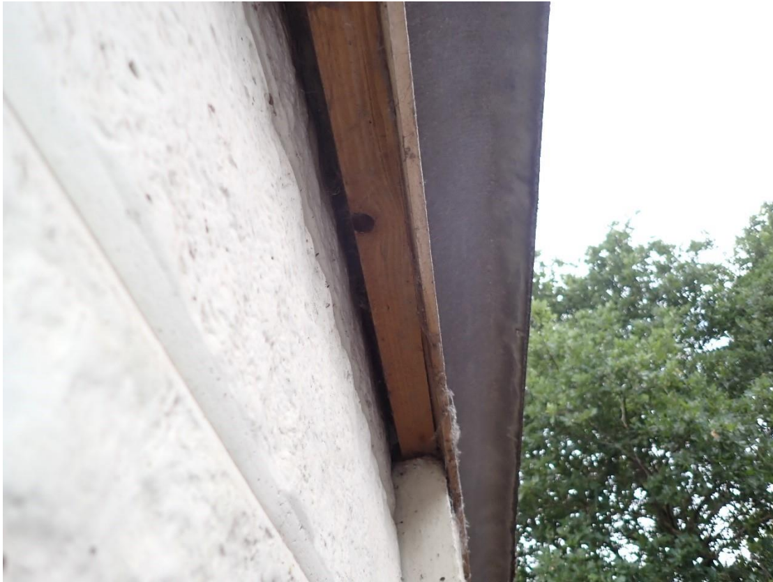
Photograph 9. Gaps underneath the barge boards on Building 1.
