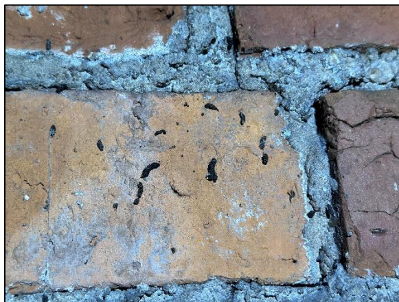
Figure 12: Bat droppings on the gable end wall.
