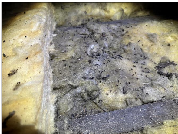
Figure 11 Bat droppings on the loft floor.
