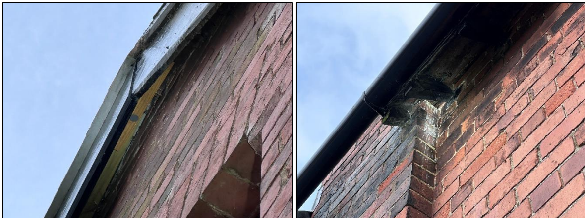
Figure 6: Voids at the gable end of the building. Figure 7: Bird droppings around voids in the eaves of the building.
