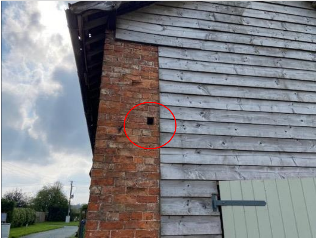
Photograph 3; A view of the brick pillars found within the infrastructure. The large gap (circled) offers an ideal entry point to a wall cavity.
