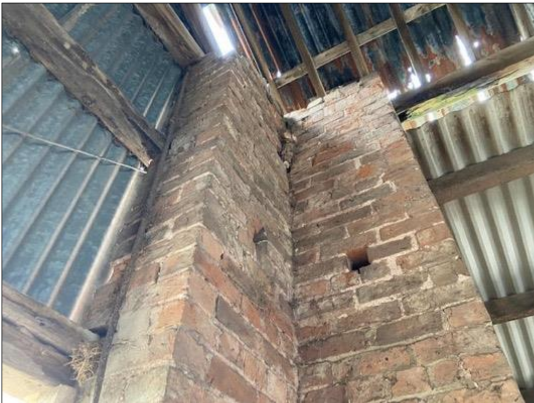
Photograph 6; A view of one of several brick pillar sections within the building. A number of openings were found across all of the brick sections, creating ideal entry points to cavities within these internal walls.
