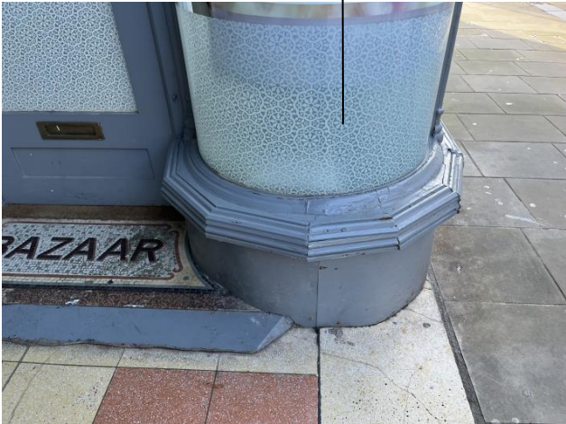
EXISTING SHOPFRONT REMOVE AND REPLACE LOW QUALITY AND DAMAGED STALLRISER
