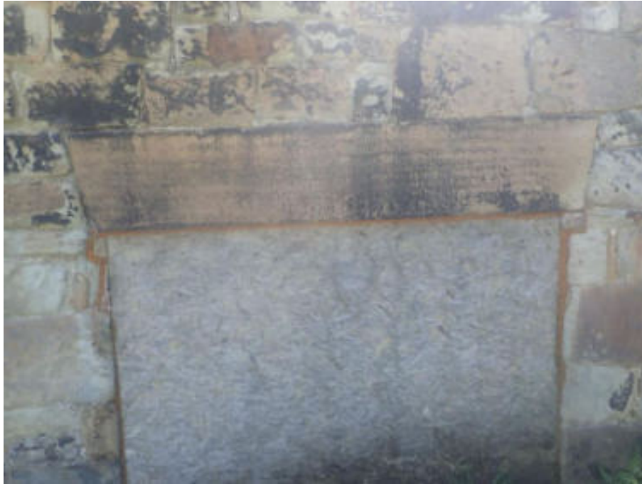
Figure 28. Failed lintel bearing
