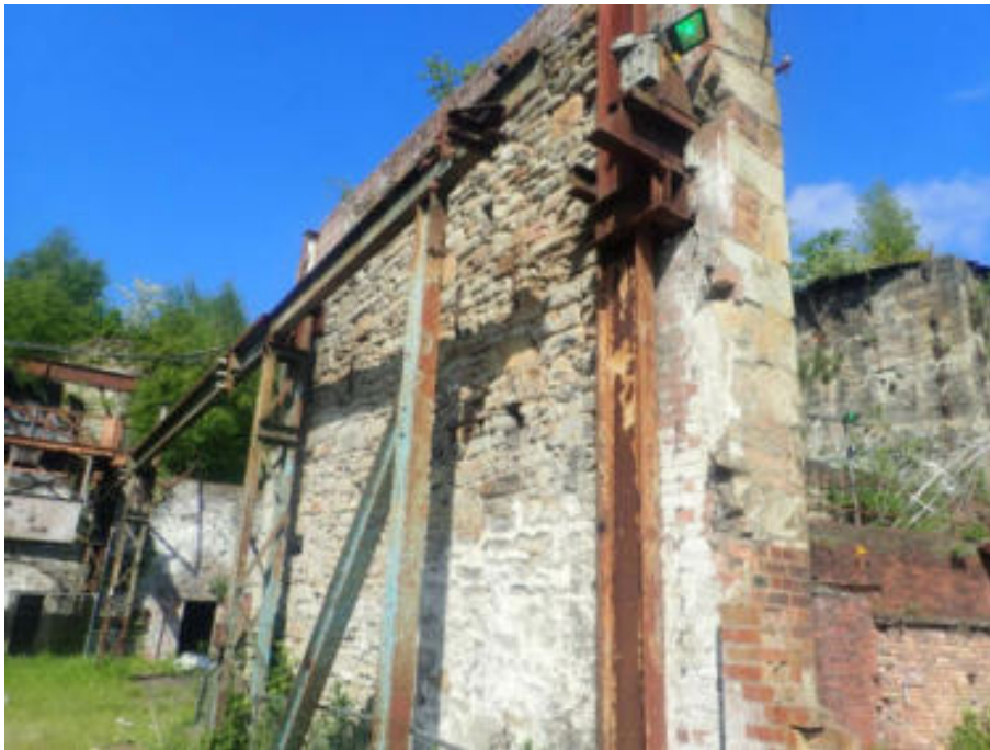
Figure 142. Spalling to brickwork
