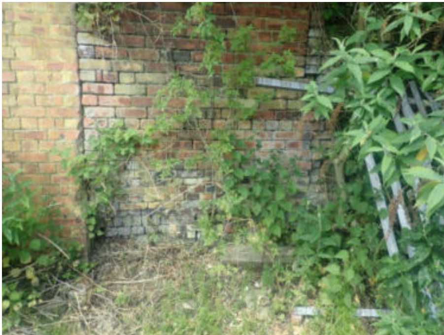
Figure 177. Typical mortar loss
