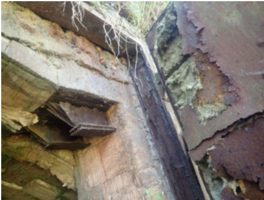
Figure 207. Deteriorated brickwork and beam
