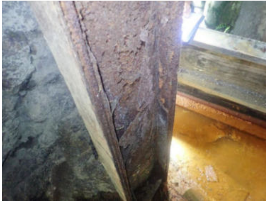
Figure 192. Corrosion to column
