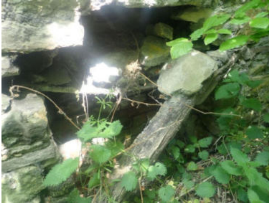
Figure 34. Failed lintel and localised collapse
