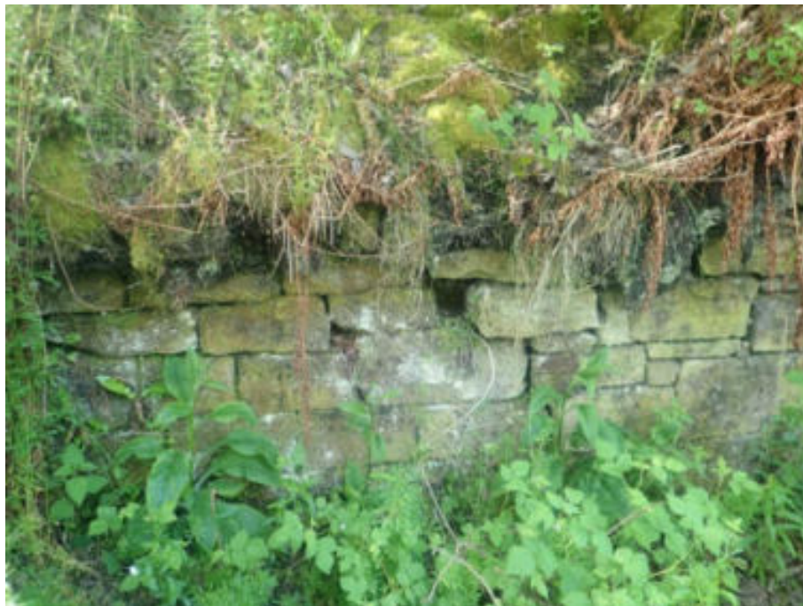
Figure 88. Typical displaced and loose masonry
