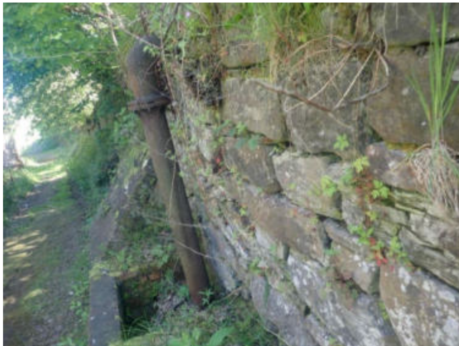
Figure 134. Bulging and leaning wall
