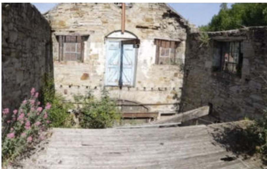
Figure 65. Failed section of 2 nd floor
