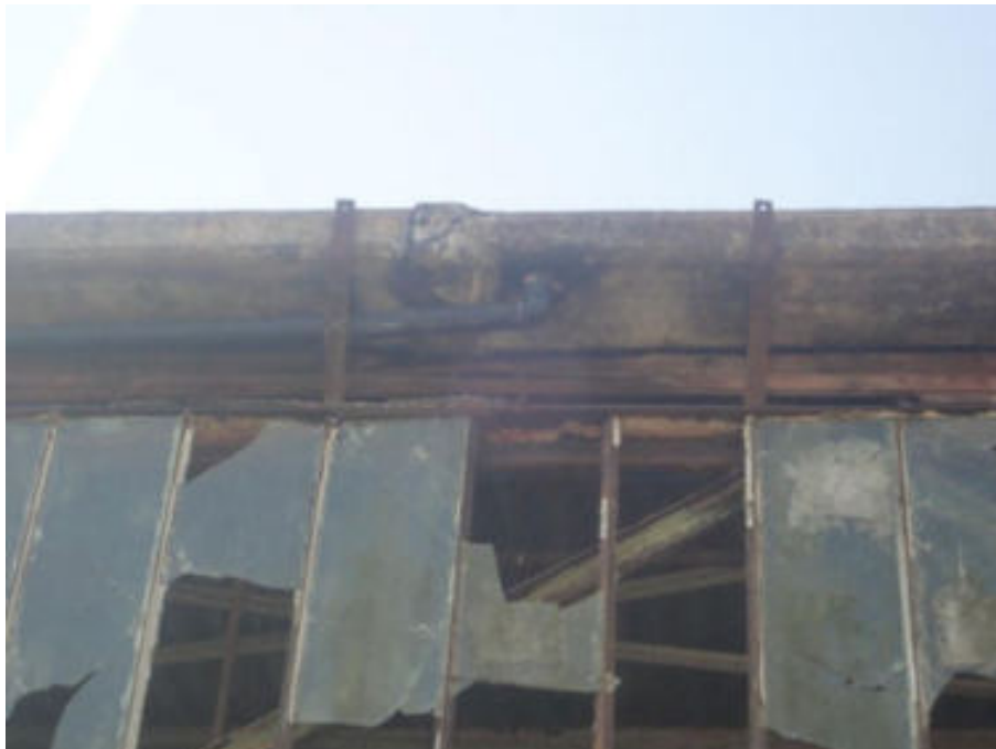
Figure 48. Typical deterioration to fascia
