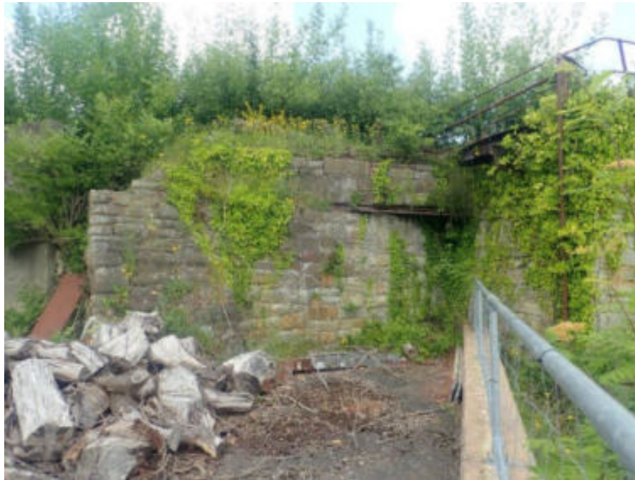
Figure 168. Corroded steel beam
