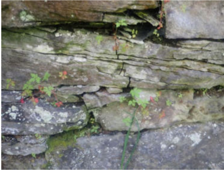
Figure 135. Typical masonry fracture
