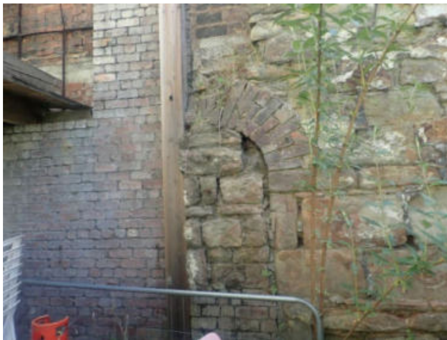
Figure 144. Typical mortar loss
