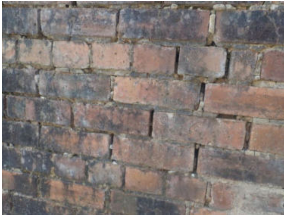
Figure 211. Typical mortar loss
