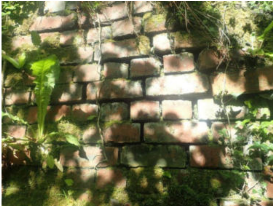
Figure 83. Typical deterioration and desiccation to pointing
