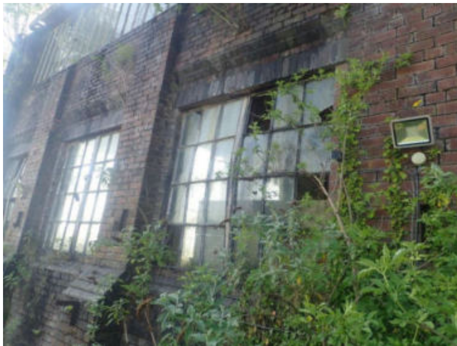
Figure 42. Corroded lintel and buckled mullion
