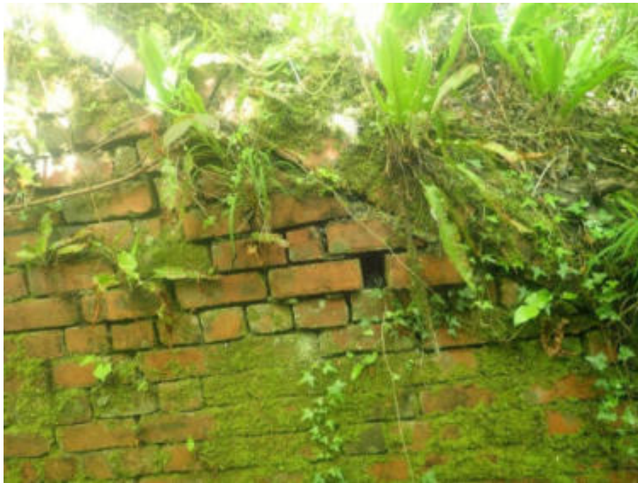
Figure 84. Area of dislodged brickwork
