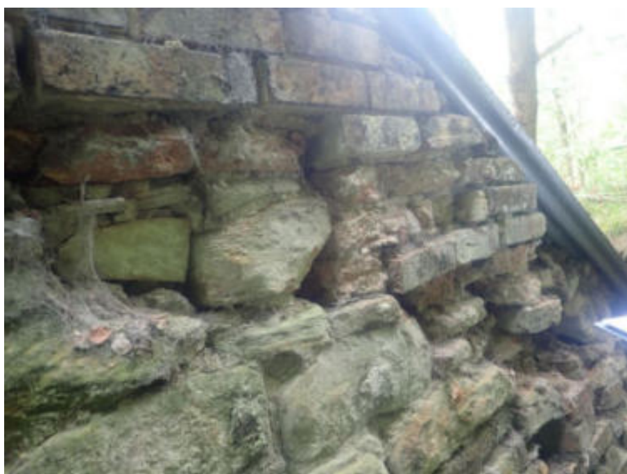
Figure 38. Failed wall panel
