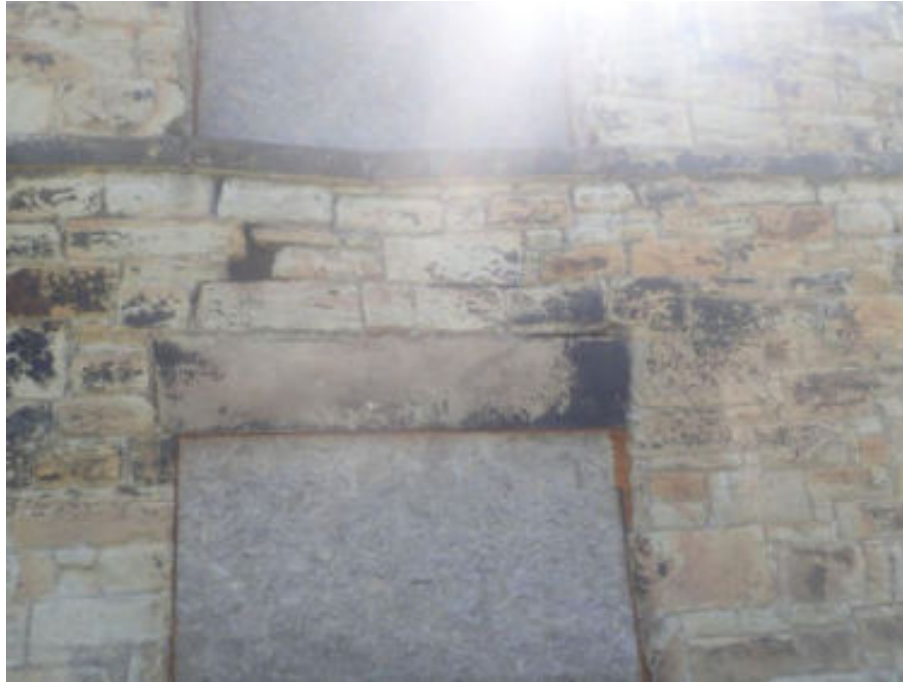
Figure 23. Failed wall panel
