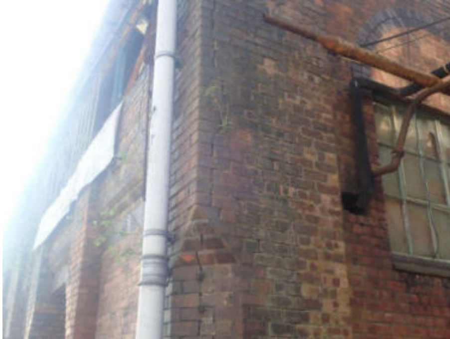
Figure 47. Typical corner fracture
