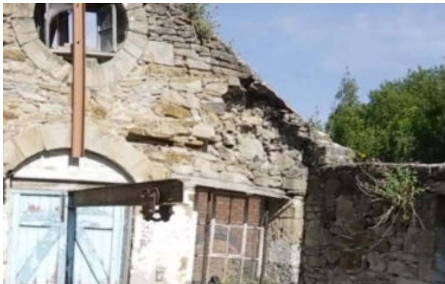
Figure 69. Localised collapse of inner leaf
