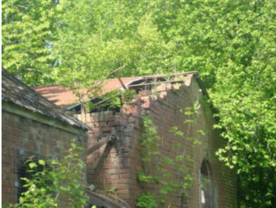
Figure 13. Failed section of roof
