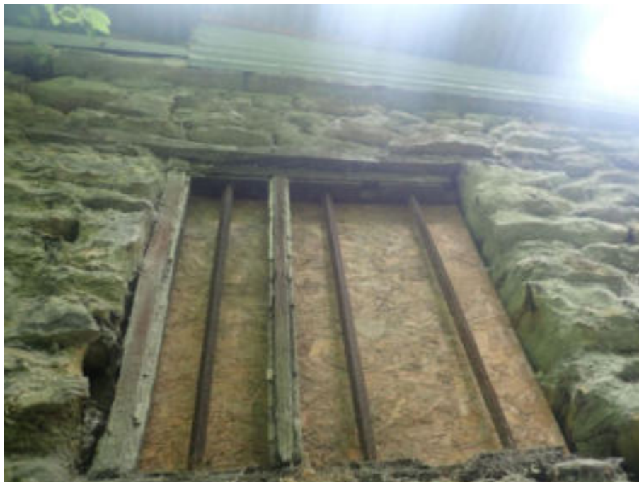
Figure 35. Failed timber lintel
