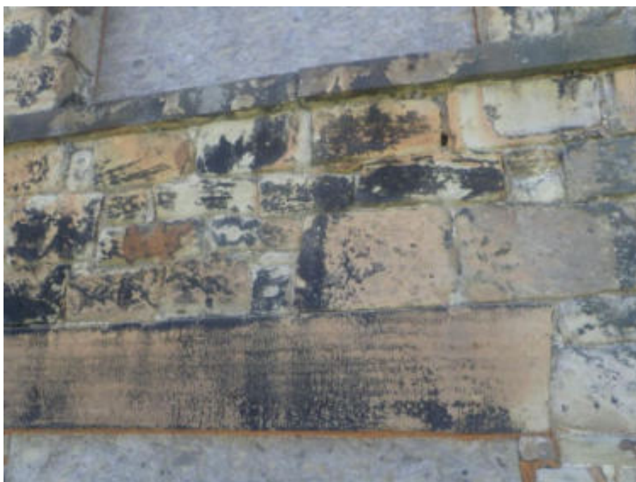
Figure 27. Failed wall panel
