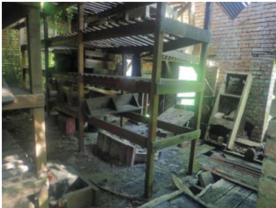
Figure 1. Typical perished timber floor covering
