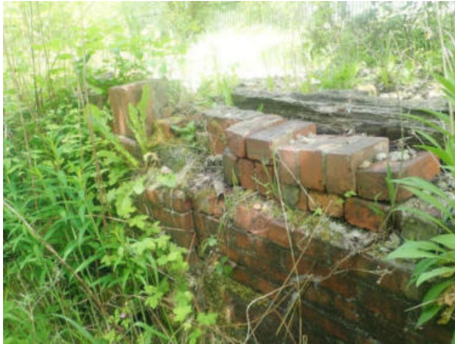
Figure 101. Typical dislodged coping
