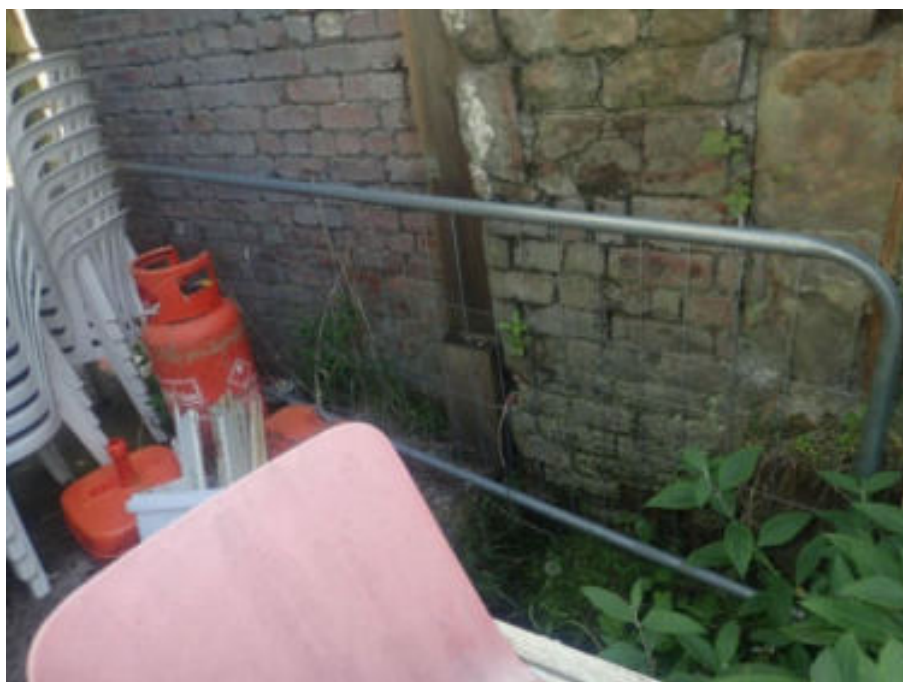
Figure 146. Typical spalling to brickwork
