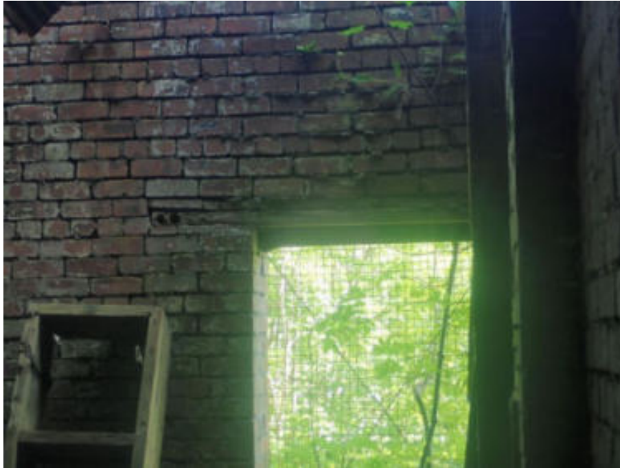
Figure 4. Typical deteriorated timber lintel
