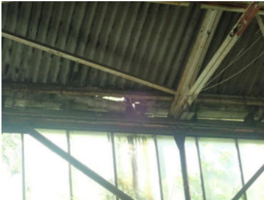
Figure 51. Corrosion to purlin
