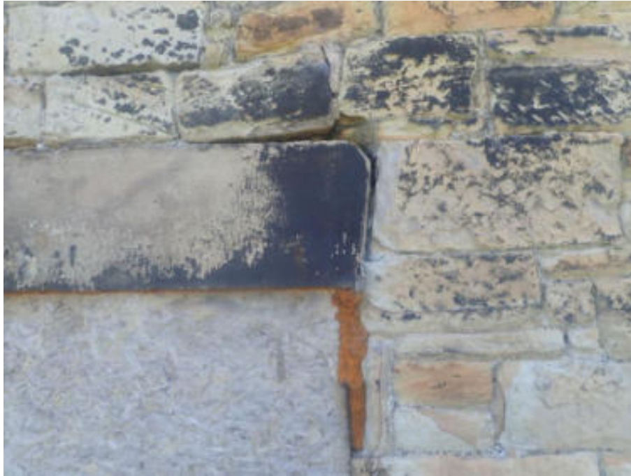
Figure 24. Failed lintel bearing
