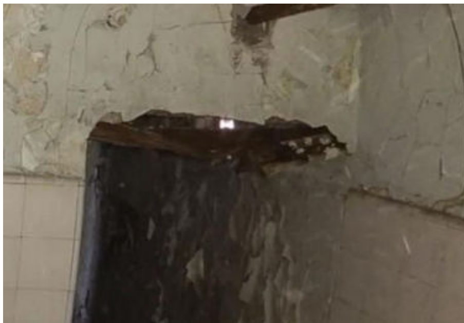
Figure 63. Typical failed lintel
