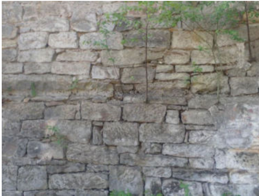
Figure 162. Typical mortar loss
