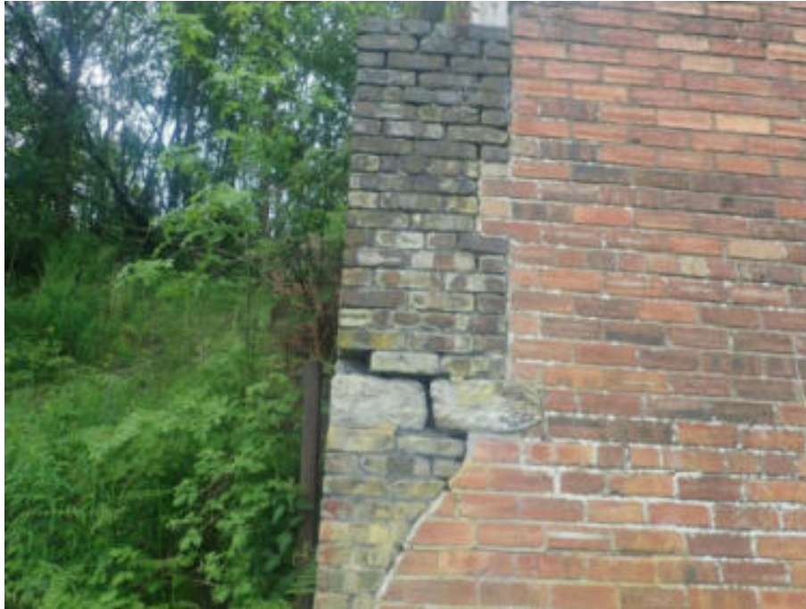
Figure 20. Insufficiently tied in infill panel
