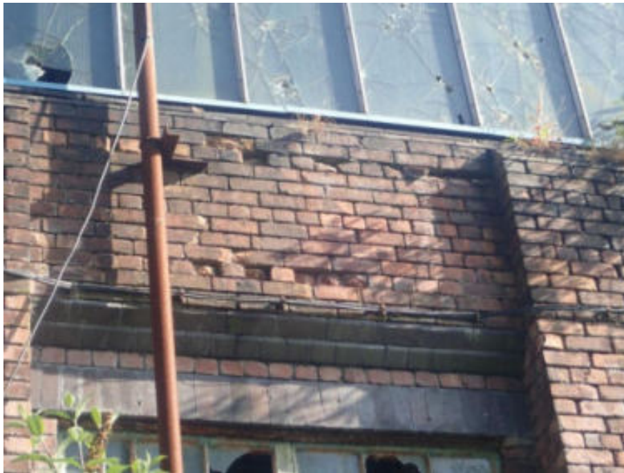
Figure 45. Typical missing and loose masonry
