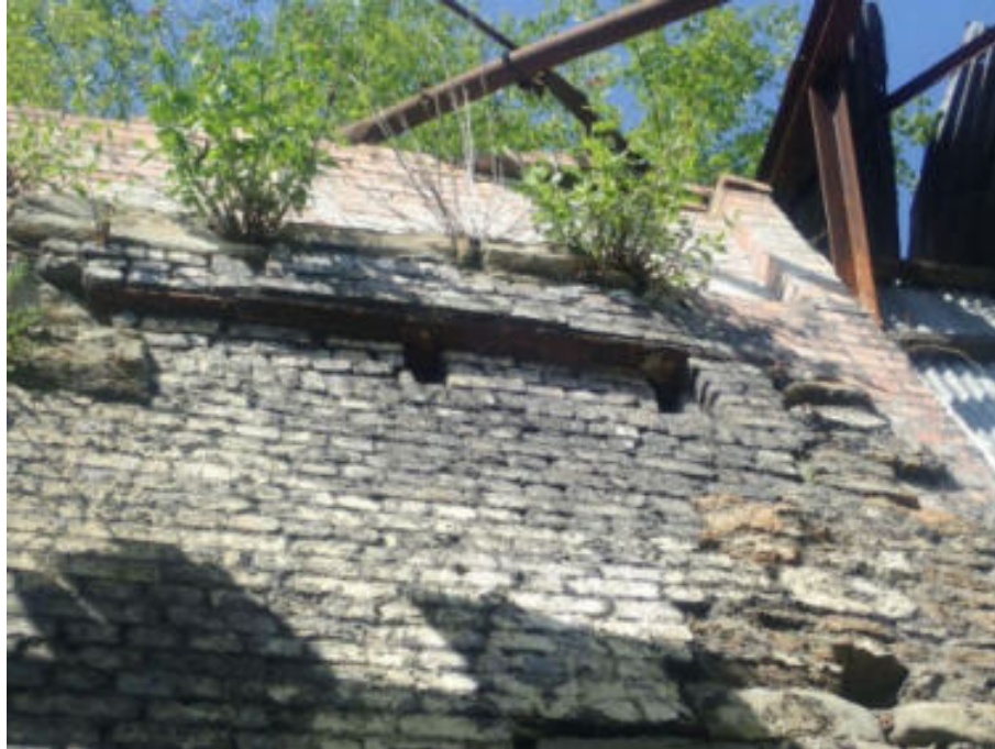
Figure 160. Typical missing masonry
