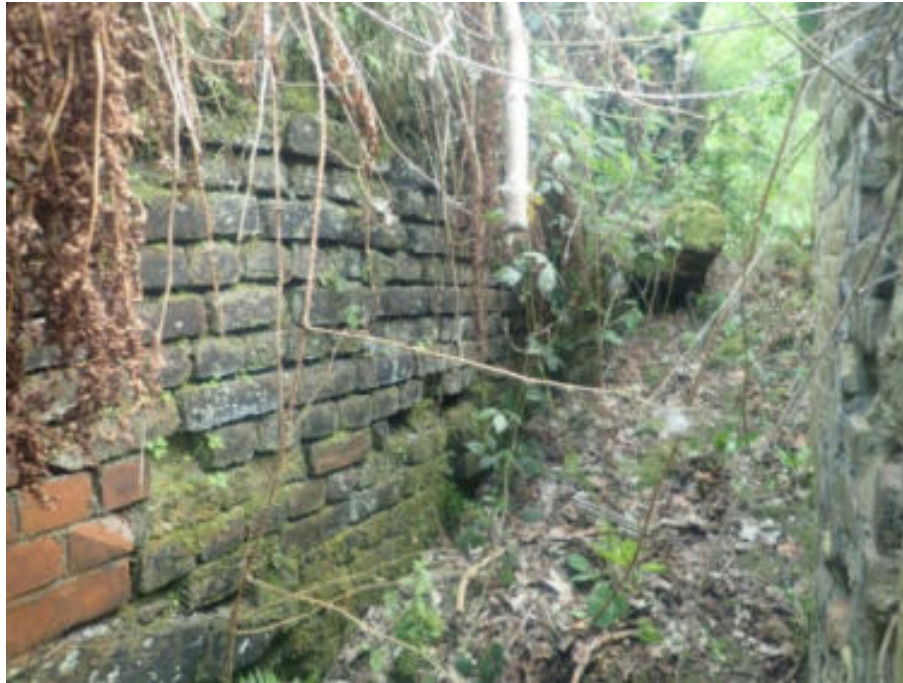
Figure 112. Debonded and dislodged brickwork
