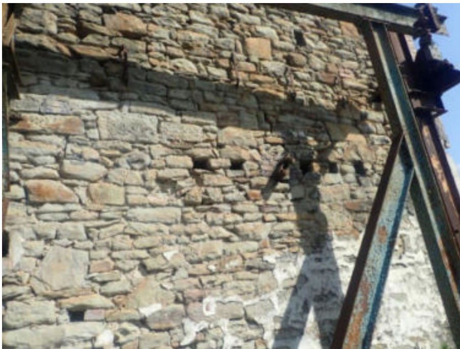
Figure 141. Missing and loose masonry
