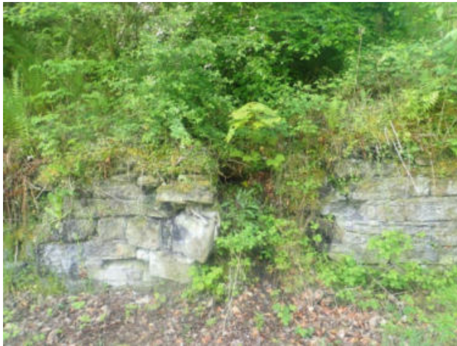
Figure 93. Failed section of wall
