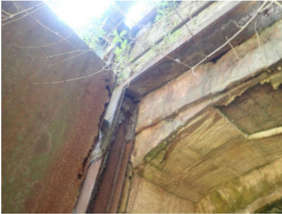
Figure 205. Corroded door frame
