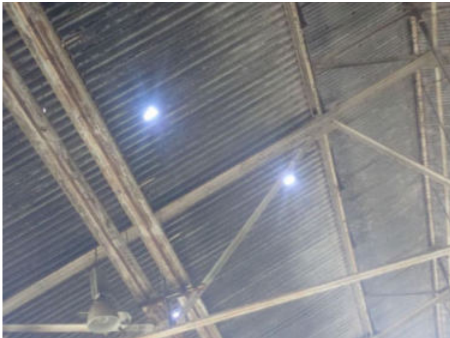
Figure 54. Typical deterioration of roof covering
