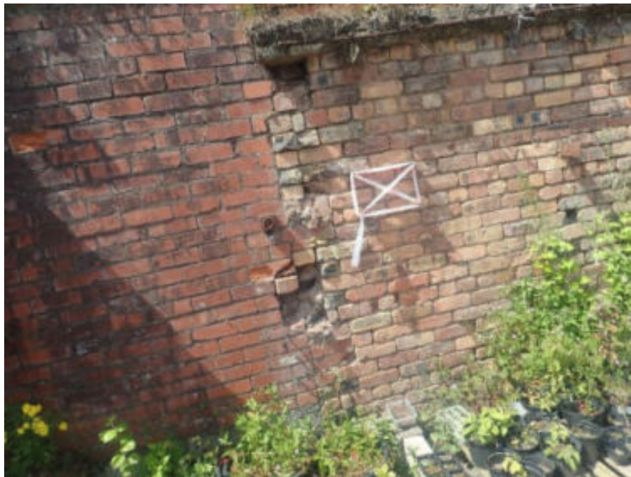
Figure 213. Typical loose and missing masonry
