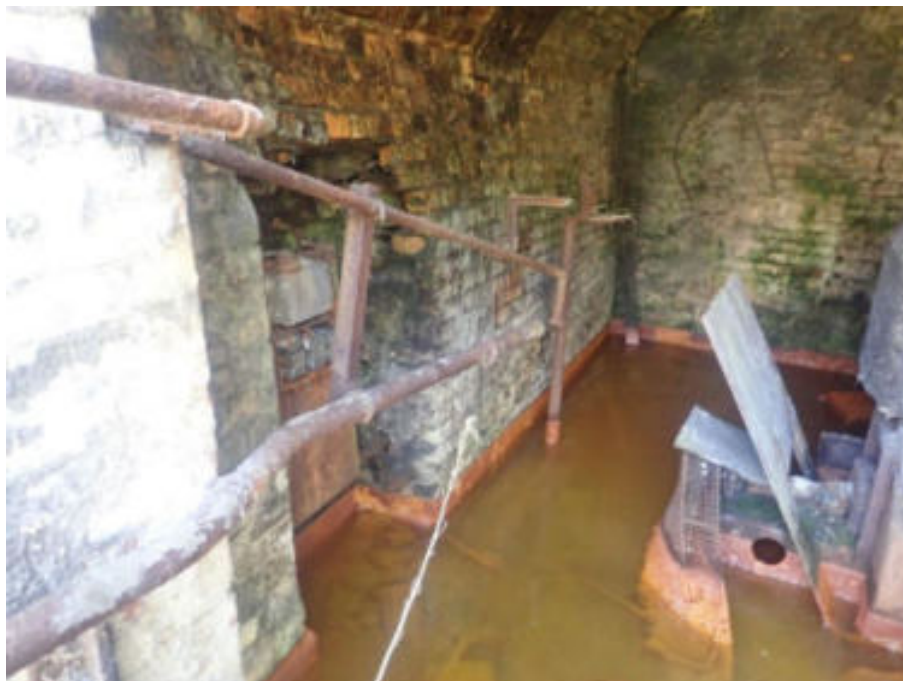
Figure 202. Typical water ingress
