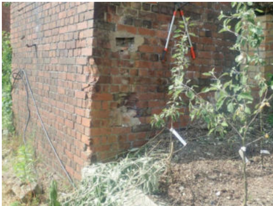
Figure 173. Typical spalled brickwork
