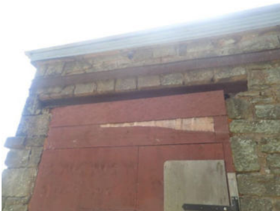
Figure 29. Insufficient bearing to stonework above lintel
