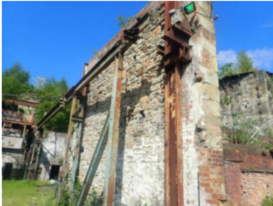
Figure 147. Spalling to brickwork
