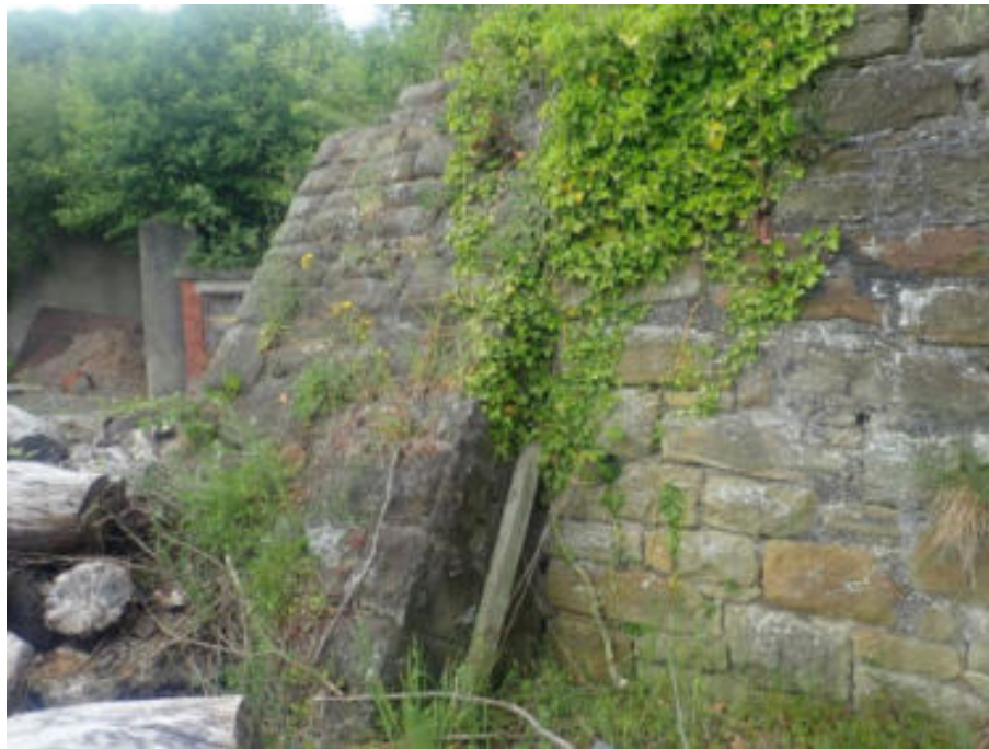
Figure 169. Typical mortar loss
