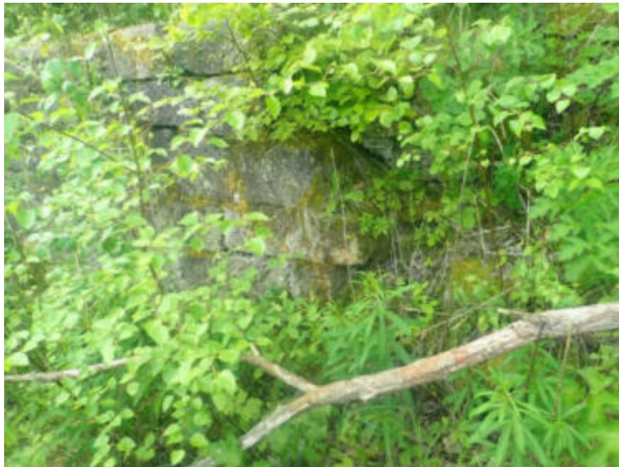
Figure 105. Typical displaced and loose masonry
