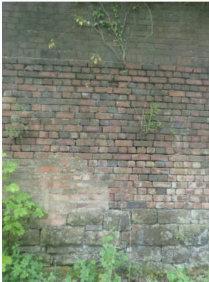
Figure 94. Typical loose and missing masonry
