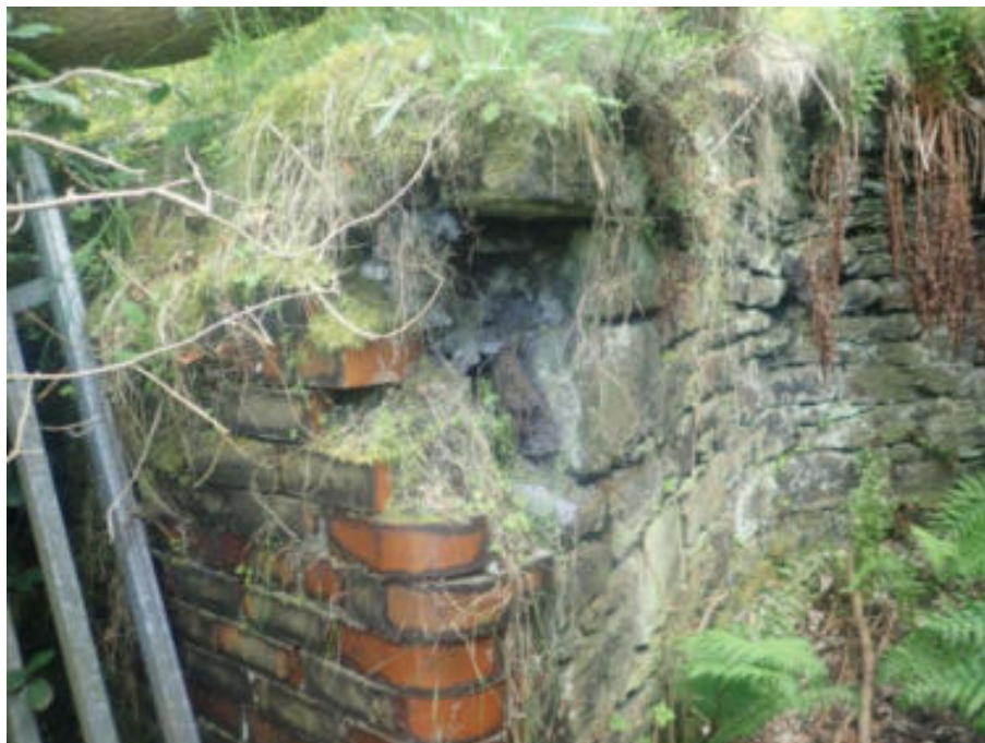
Figure 111. Partially collapsed wall
