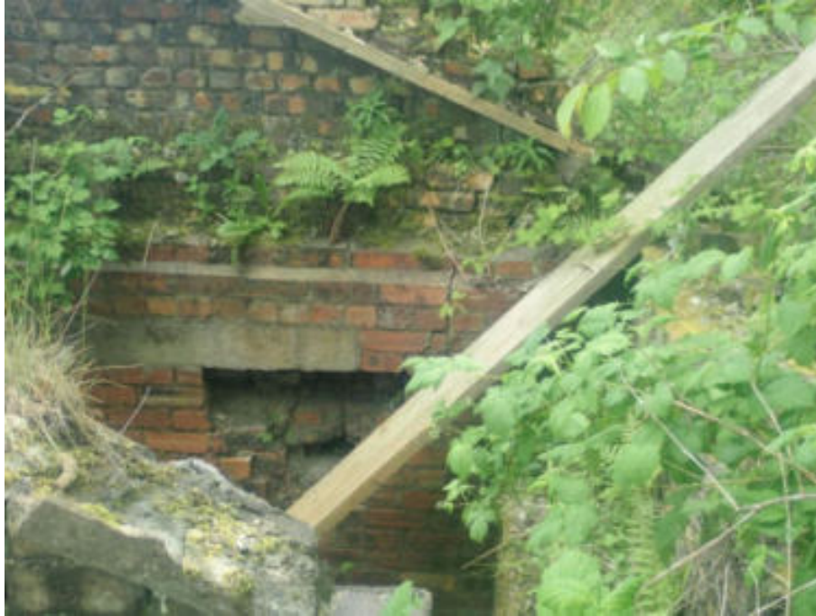
Figure 19. Vertical stress fracture
