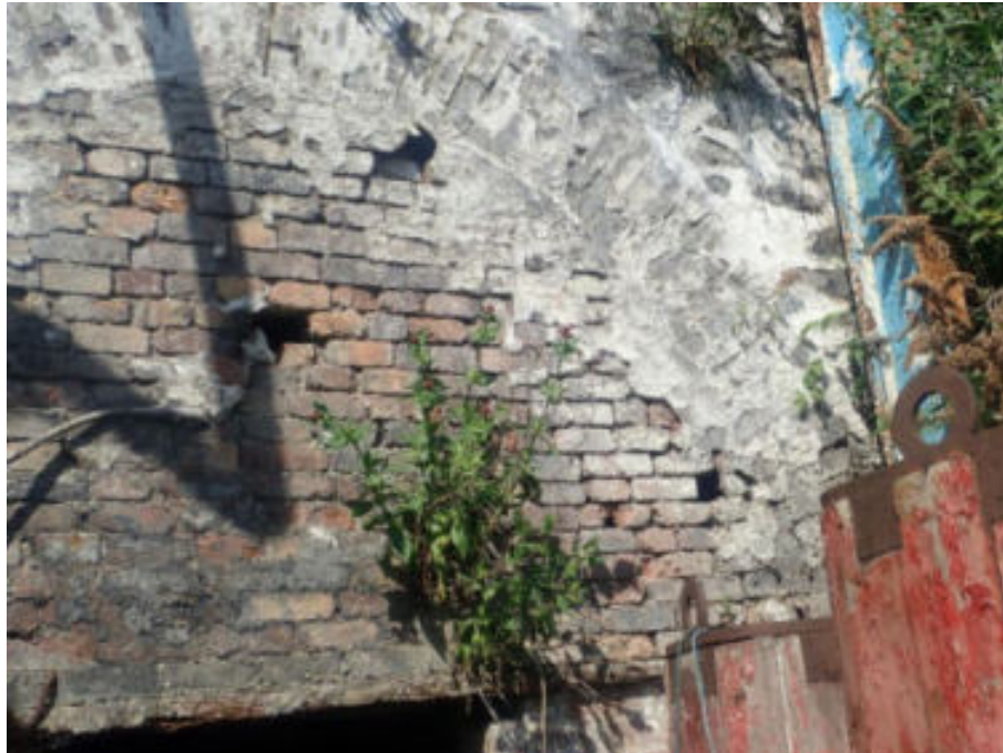
Figure 155. Typical missing masonry
