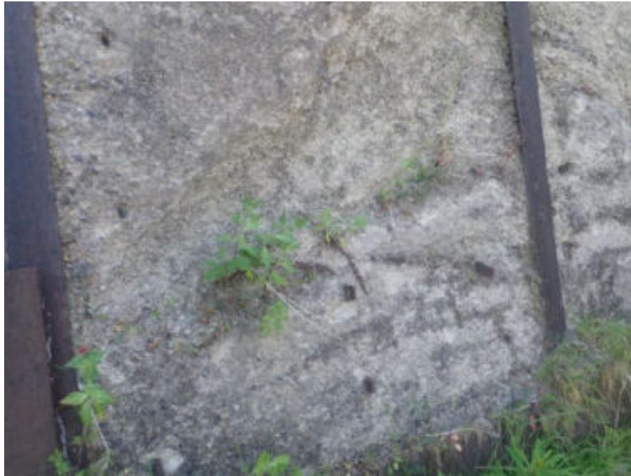
Figure 129. Typical concrete scaling
