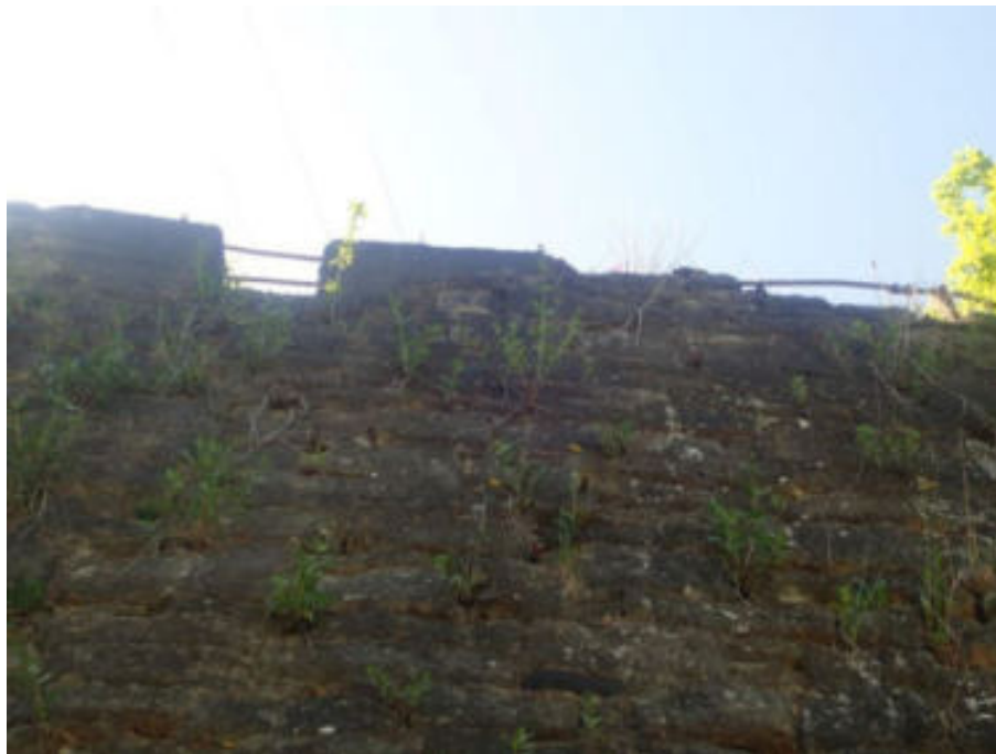
Figure 131. Typical mortar loss
