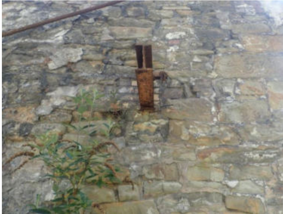
Figure 145. Typical corrosion to steel
