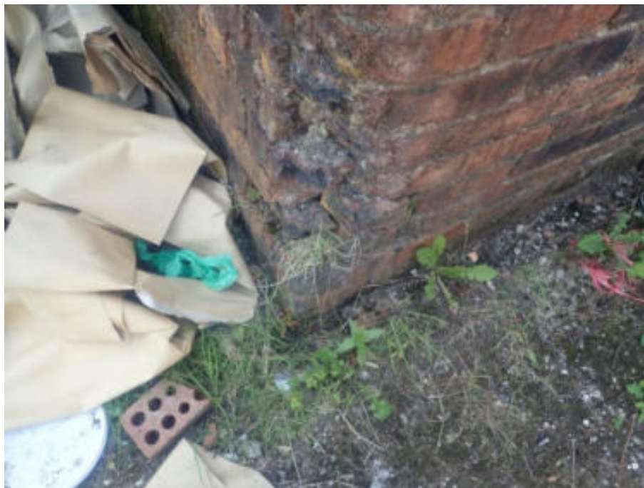
Figure 212. Typical spalled brickwork
