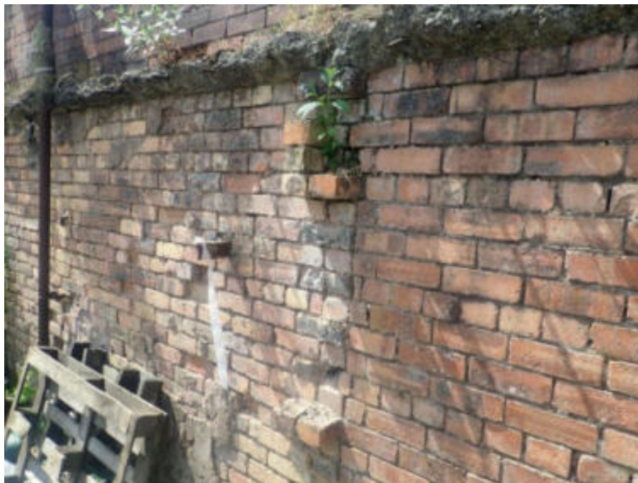
Figure 215. Typical missing mortar
