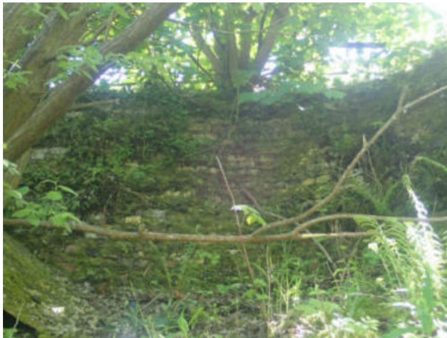
Figure 124. General view of wall showing mortar loss, vegetation growth and tree
