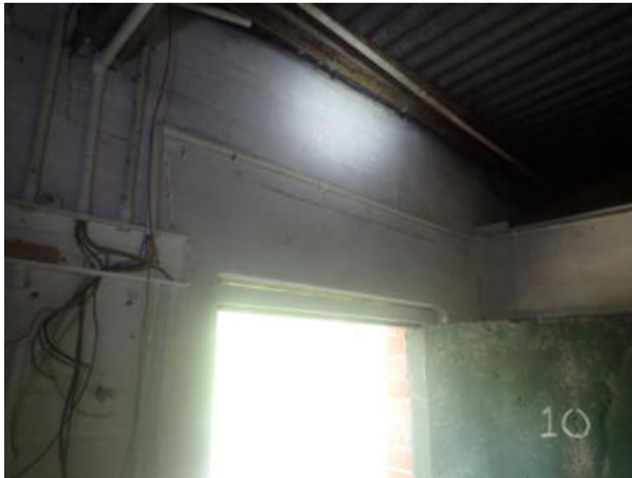
Figure 217. Typical cracking above lintel
