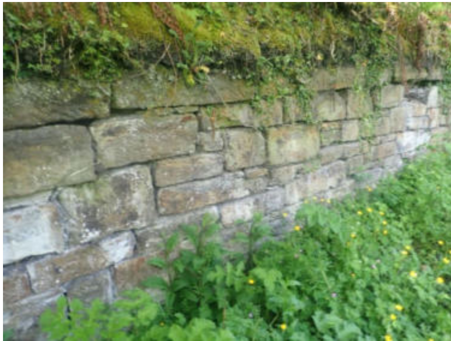
Figure 89. Typical mortar loss
