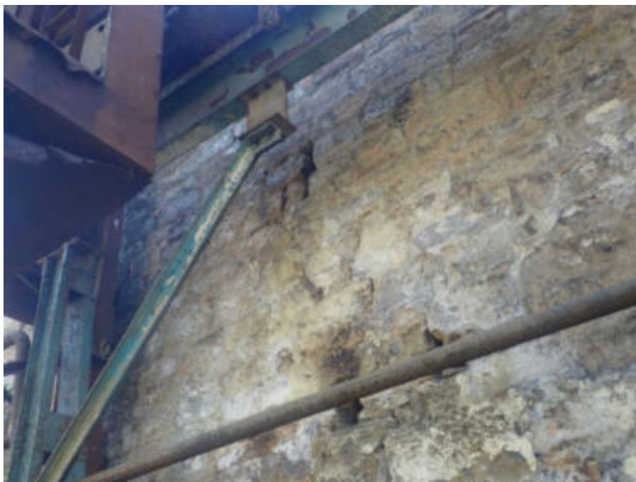
Figure 61. Typical missing masonry
