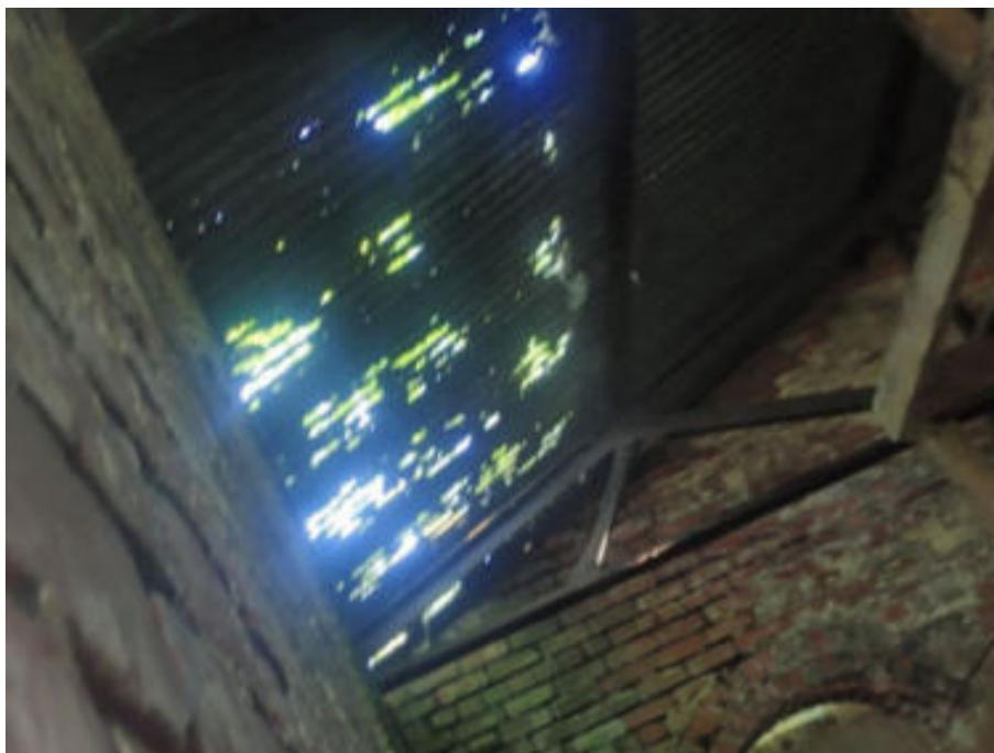
Figure 3. Typical corrosion to corrugated profile steel roof
