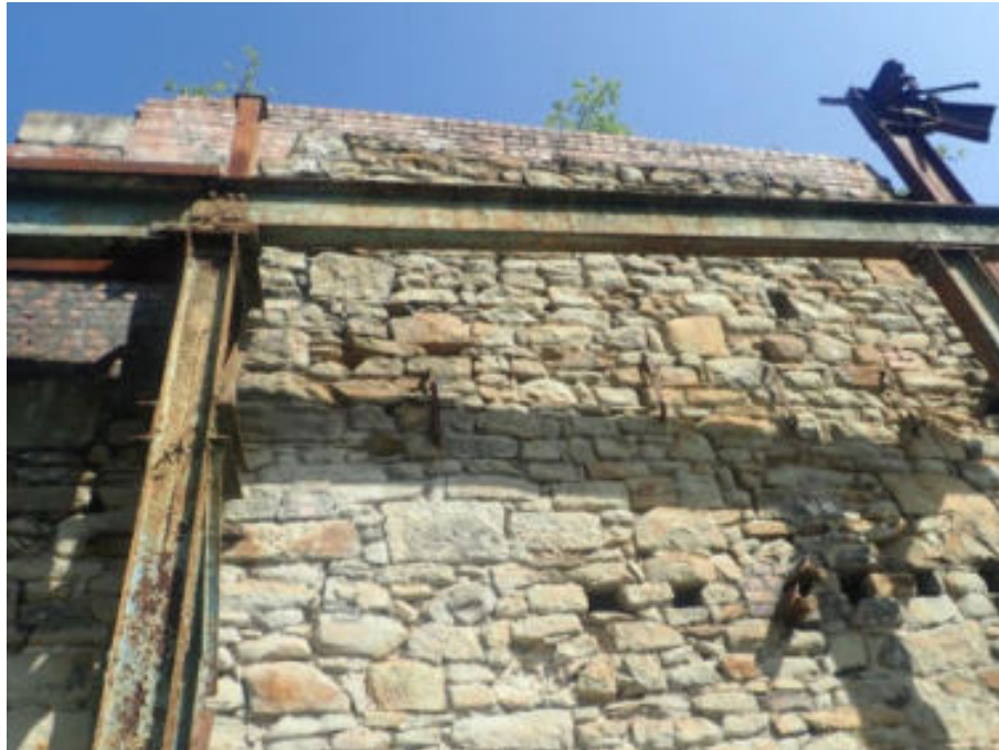
Figure 139. Typical mortar loss
