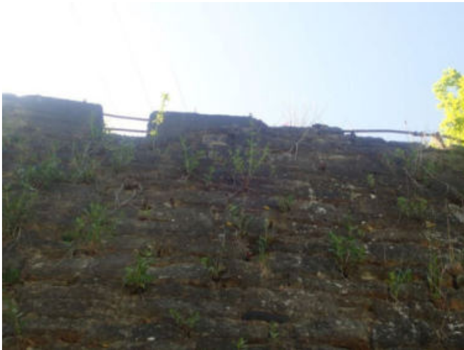
Figure 133. Dislodged and missing masonry
