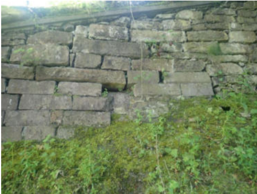
Figure 137. Dislodged and missing masonry
