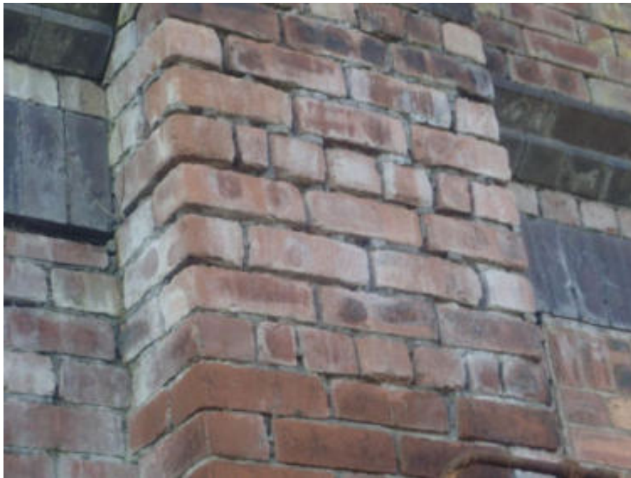
Figure 49. Typical desiccated mortar
