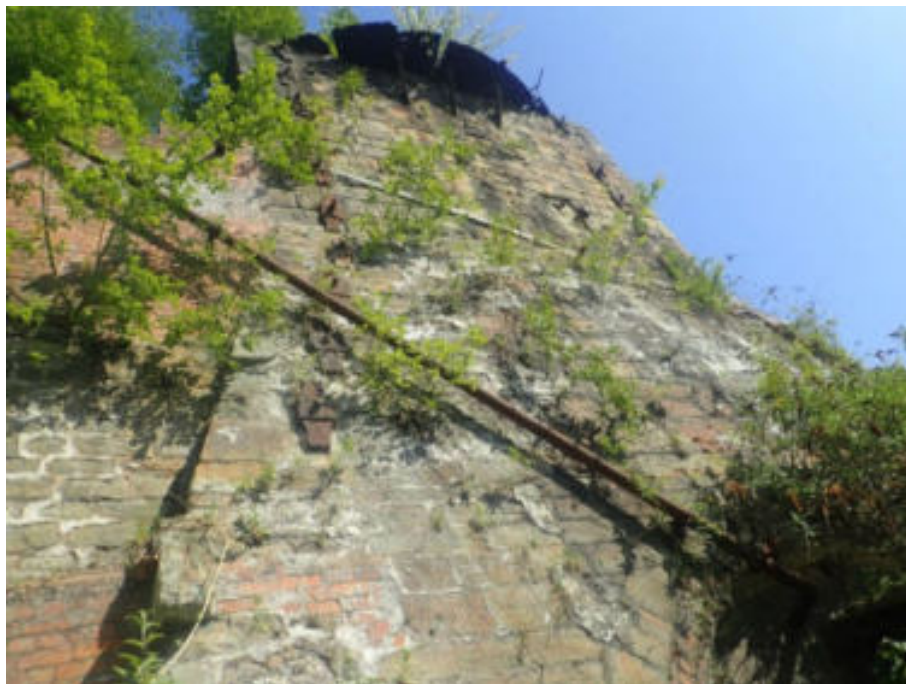
Figure 75. Typical mortar loss
