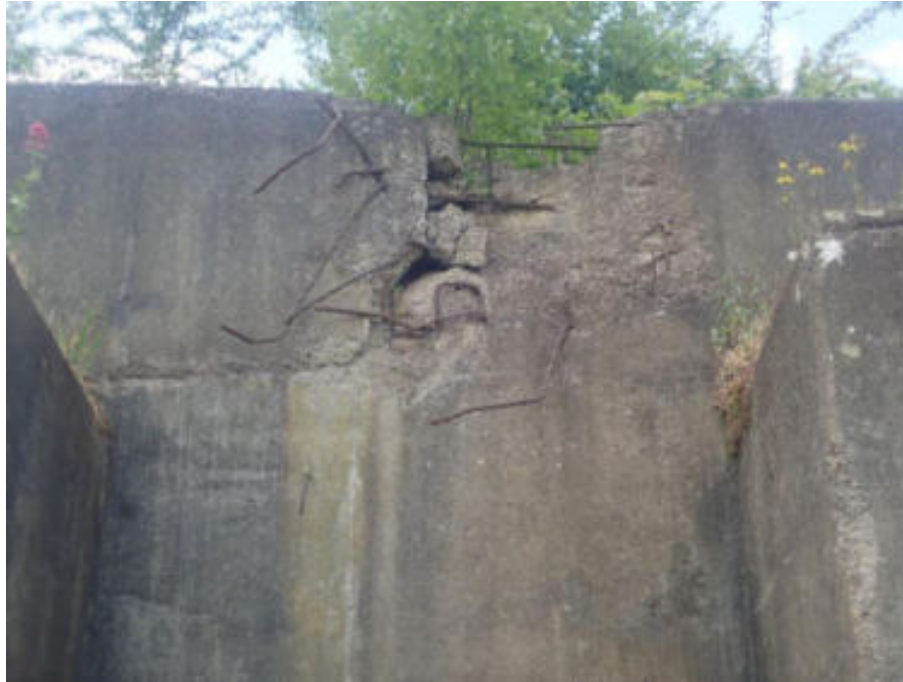
Figure 165. Failed area of wall
