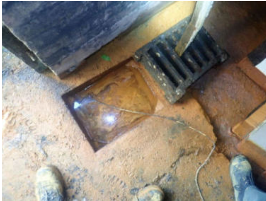
Figure 188. Debris in gully
