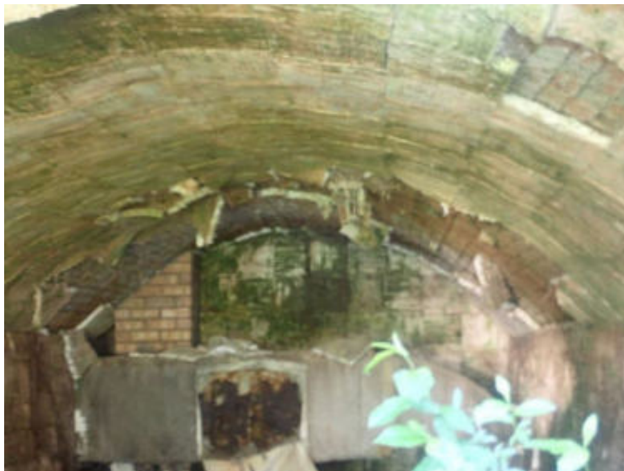
Figure 204. Deterioration to plasterboard
