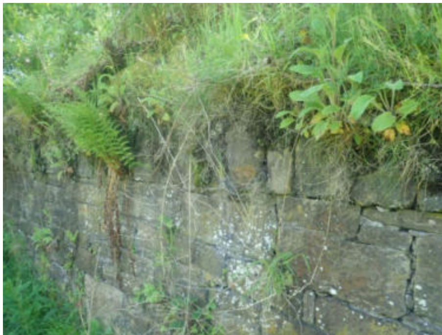
Figure 118. Typical loose copings
