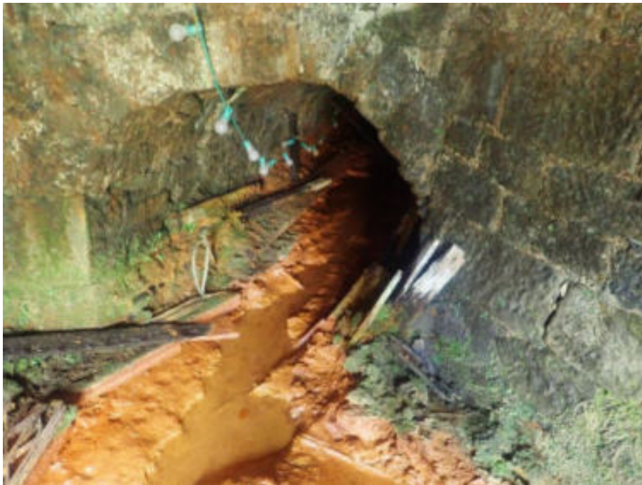
Figure 196. Typical mortar loss
