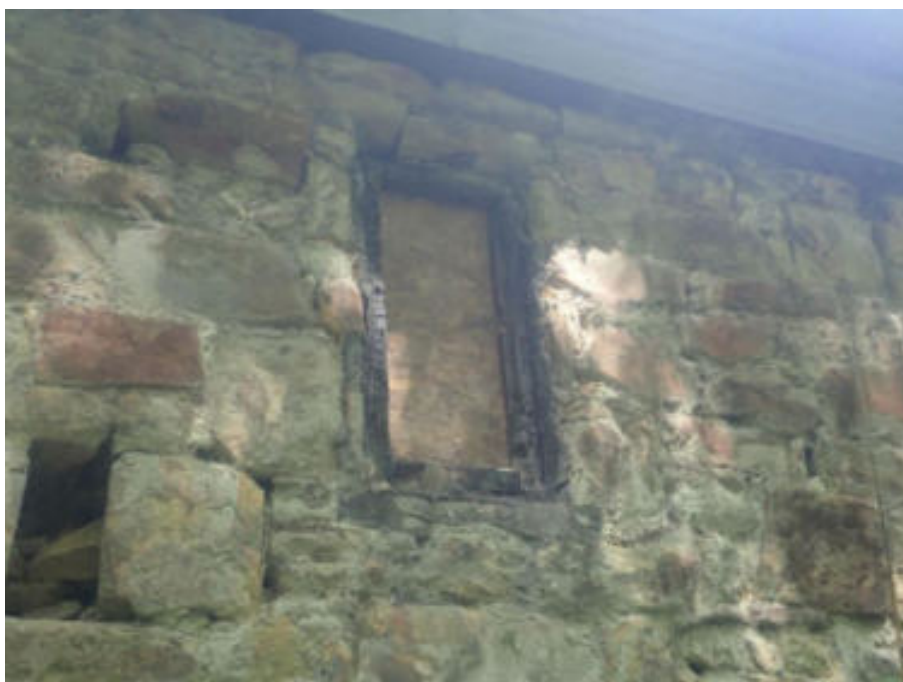
Figure 33. Fire damaged window frame
