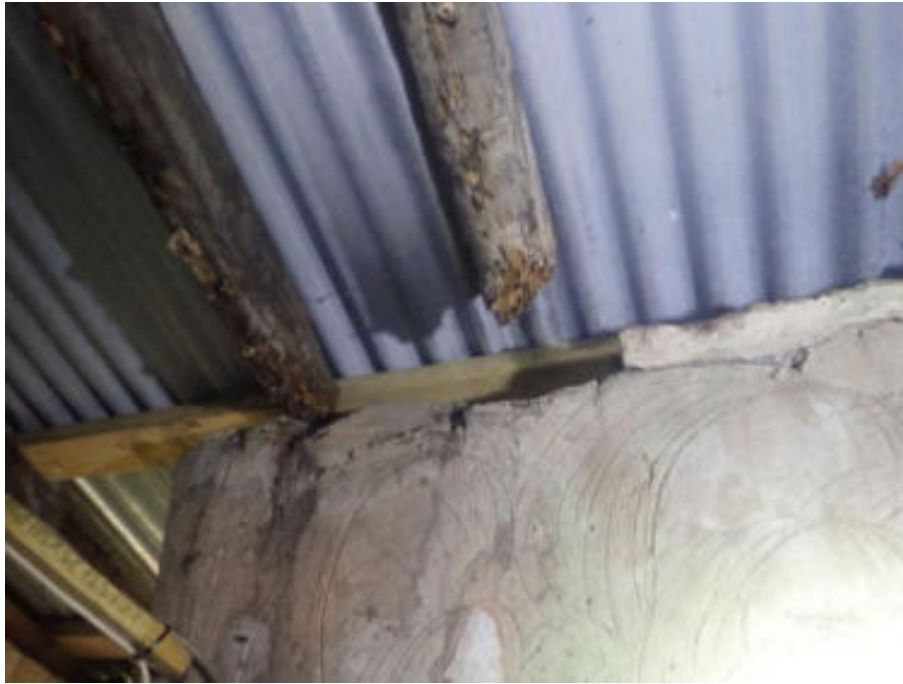
Figure 40. Typical loss of fixity
