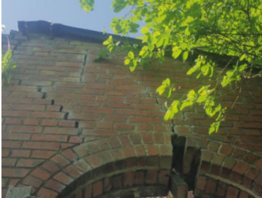
Figure 12. Failed masonry arch
