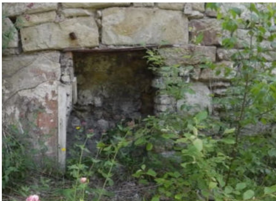
Figure 67. Deflection to lintel
