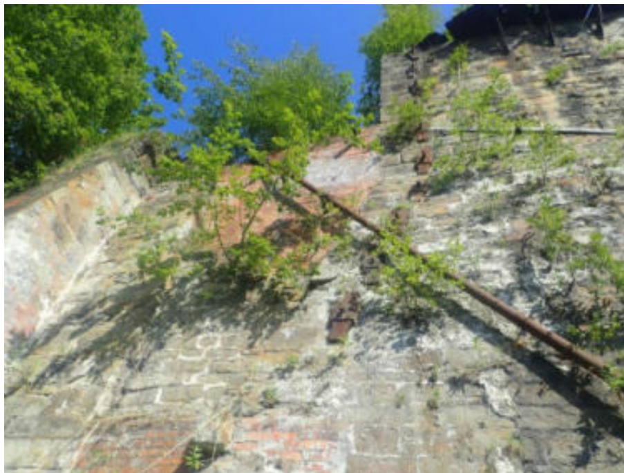
Figure 153. Typical mortar loss
