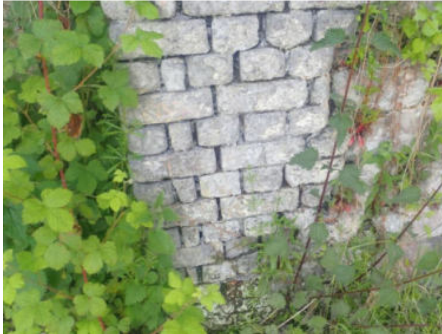
Figure 156. Typical mortar loss
