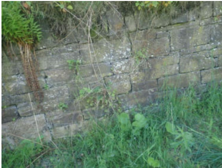
Figure 117. Typical mortar loss
