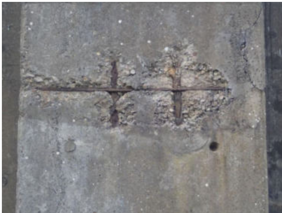
Figure 164. Exposed and corroded bars
