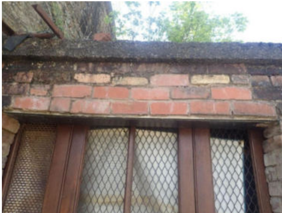
Figure 210. Deflection to lintel
