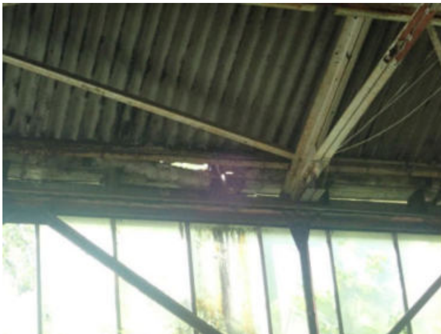
Figure 56. Typical corrosion to truss
