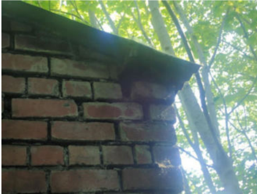
Figure 8. Typical dislodged brickwork on corner
