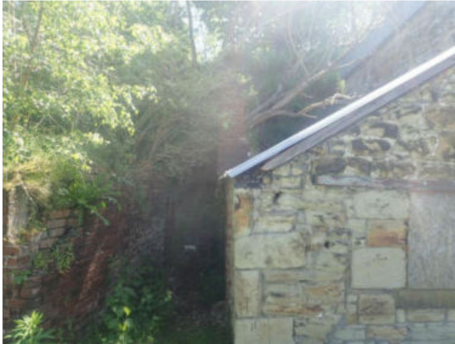
Figure 39. Significant outward lean in stack
