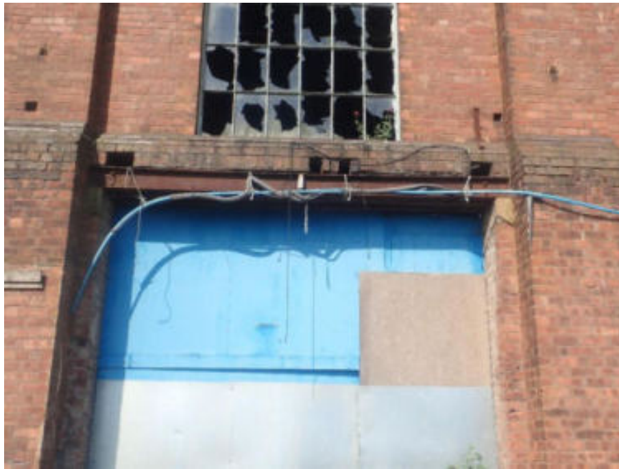
Figure 43. Deflected and corroded lintel
