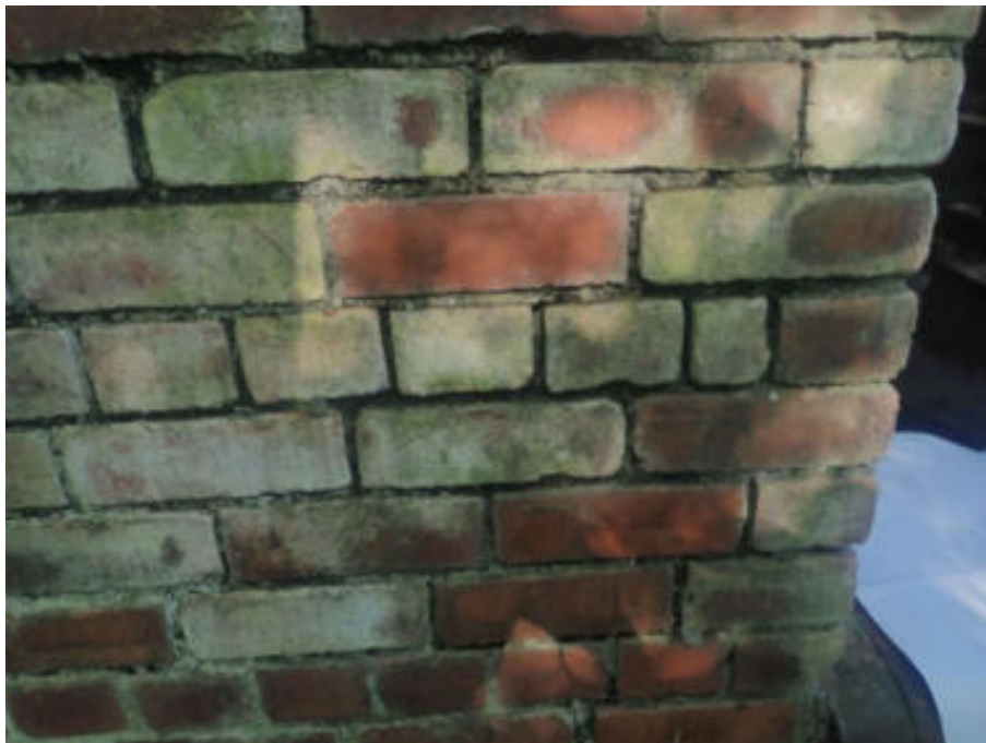
Figure 7. Typical desiccated mortar pointing
