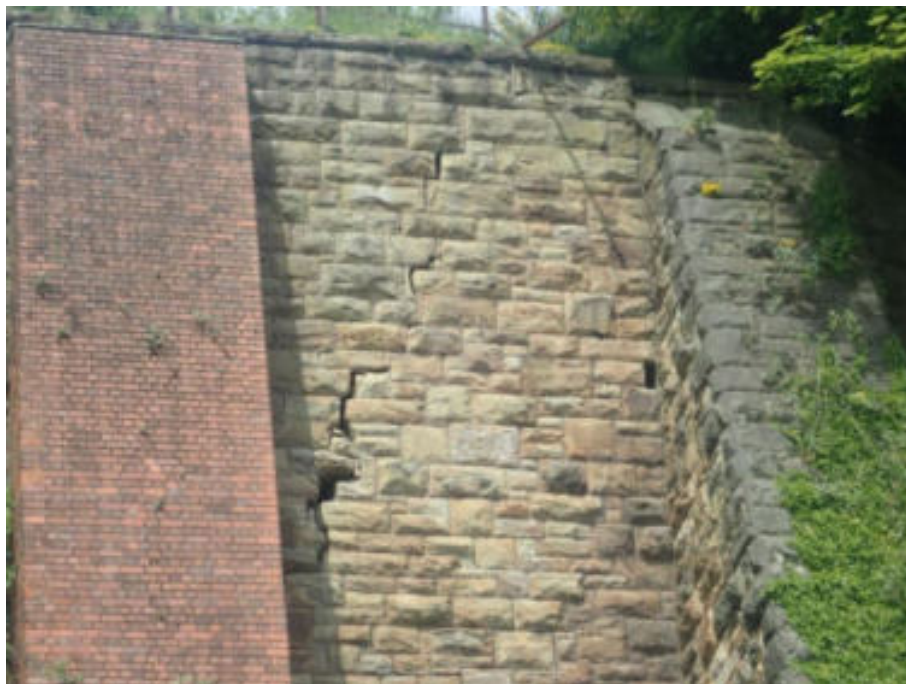
Figure 175. Typical missing and loose masonry
