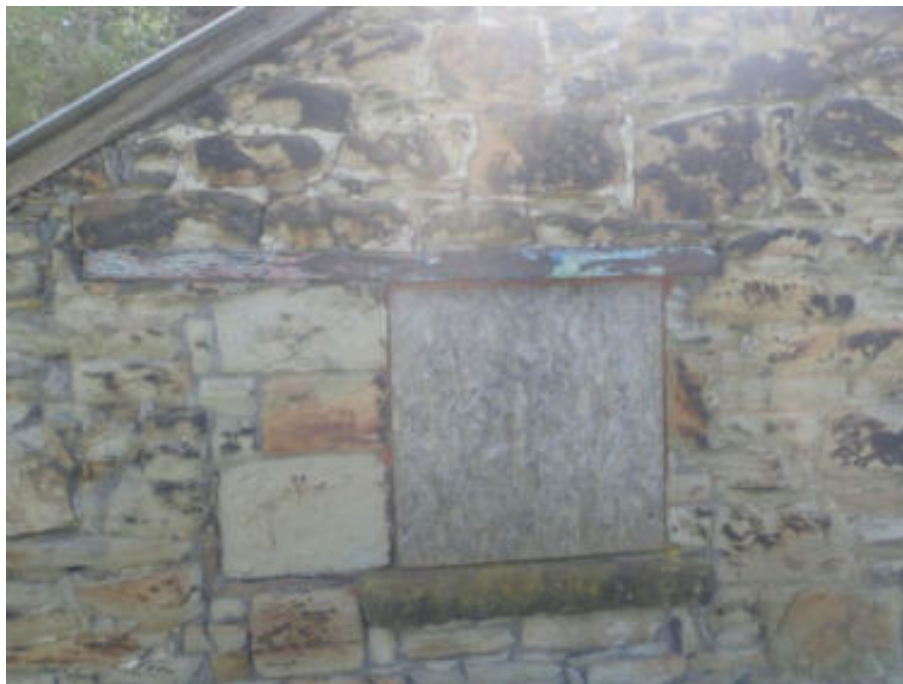
Figure 22. Deteriorated timber lintel
