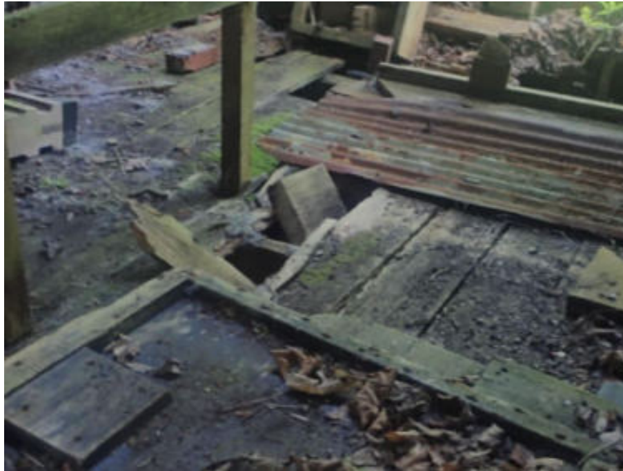
Figure 2. Typical deteriorated floor joists
