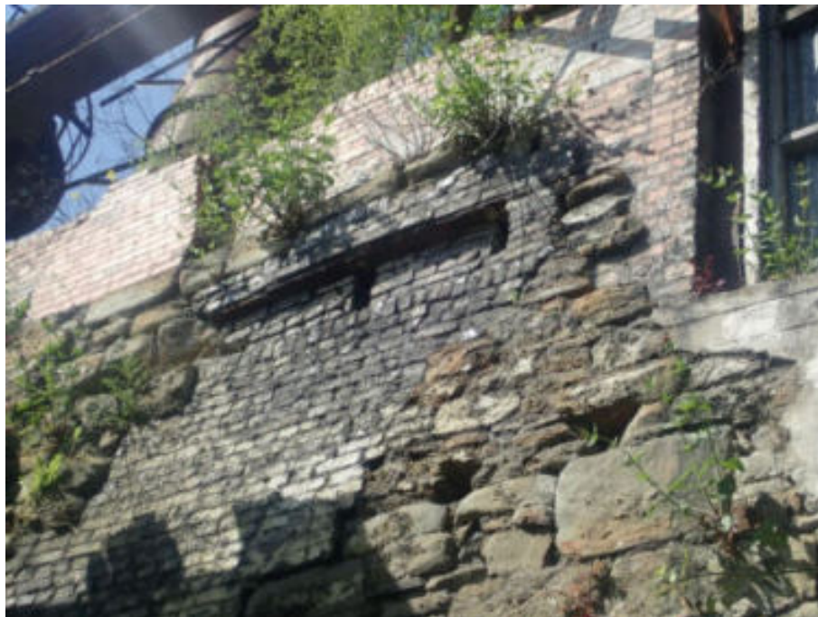
Figure 159. Typical mortar loss
