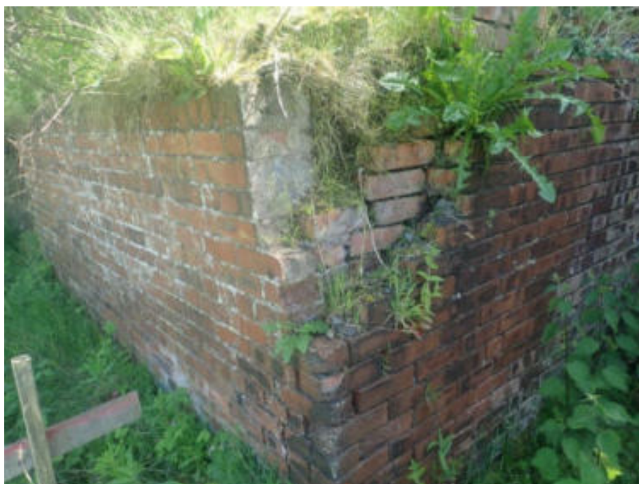
Figure 113. Leaning section of wall
