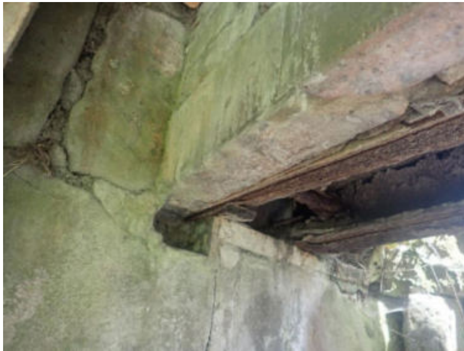
Figure 151. Corroded PFCs and unsupported blockwork
