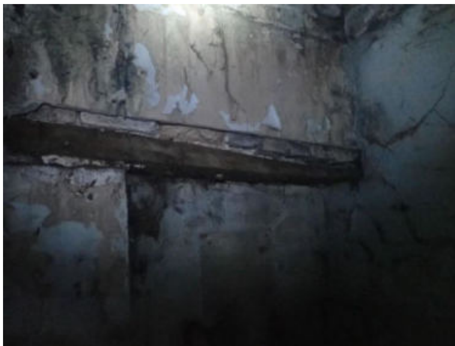
Figure 41. Inadequate timber lintel
