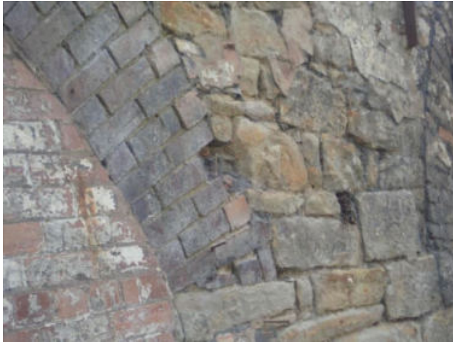
Figure 149. Typical missing masonry
