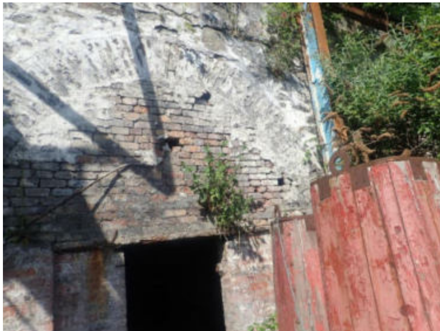
Figure 157. Typical weathered render
