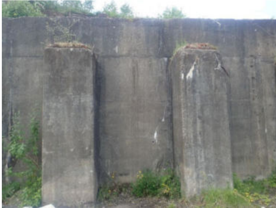
Figure 167. Typical staining on wall
