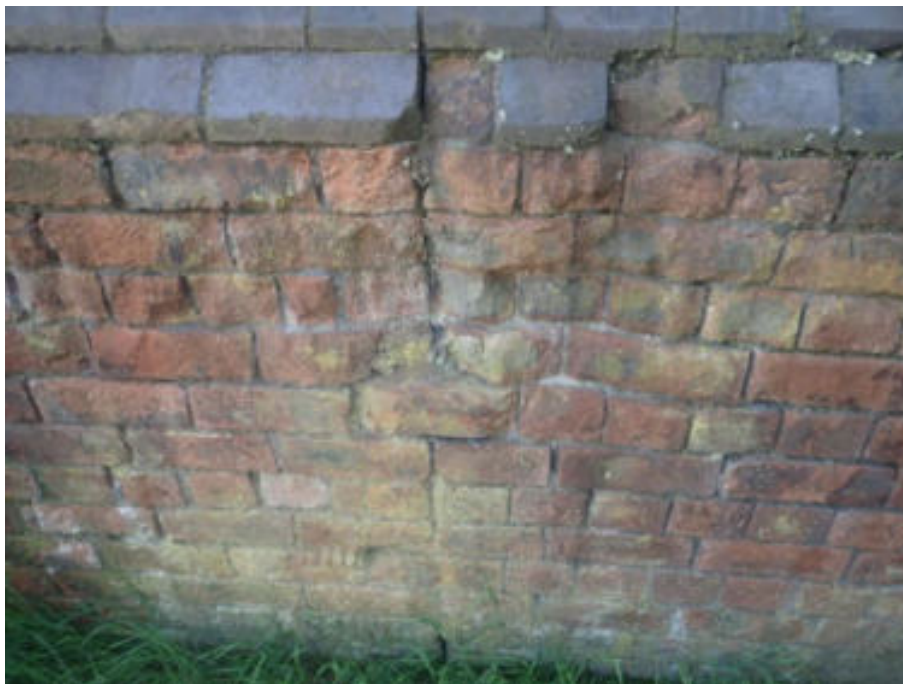
Figure 46. Typical deteriorated brickwork
