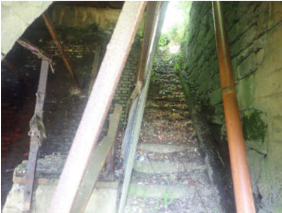
Figure 193. Debris on stairs
