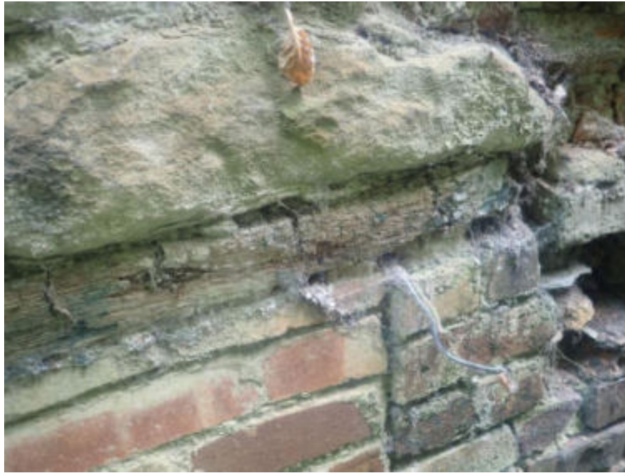
Figure 37. Failed timber lintel
