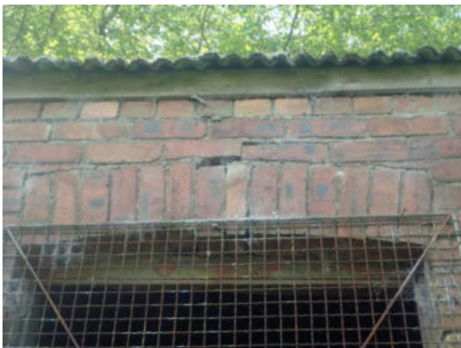
Figure 15. Failed masonry arch
