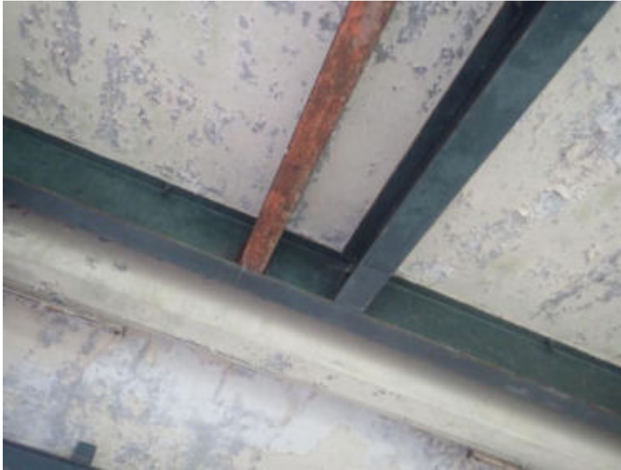
Figure 221. Typical corrosion to beam
