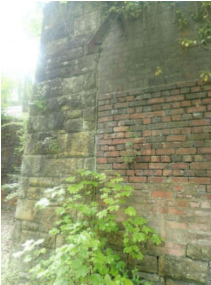
Figure 95. Typical mortar loss
