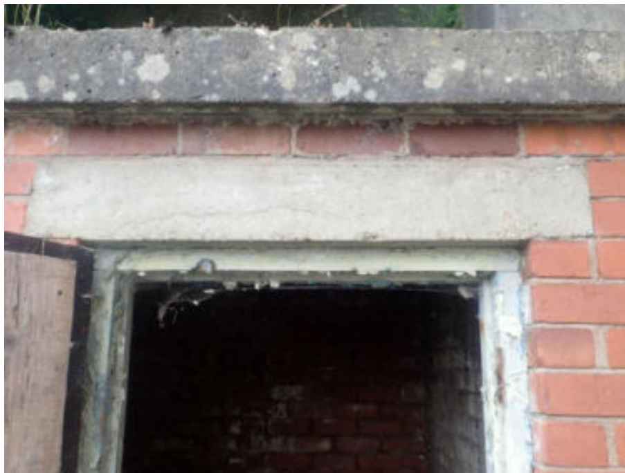
Figure 220. Deflected and cracked lintel
