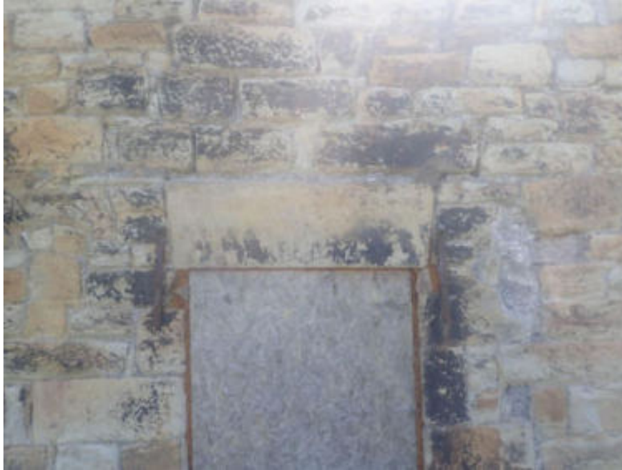
Figure 25. Historical failure to lintel bearing
