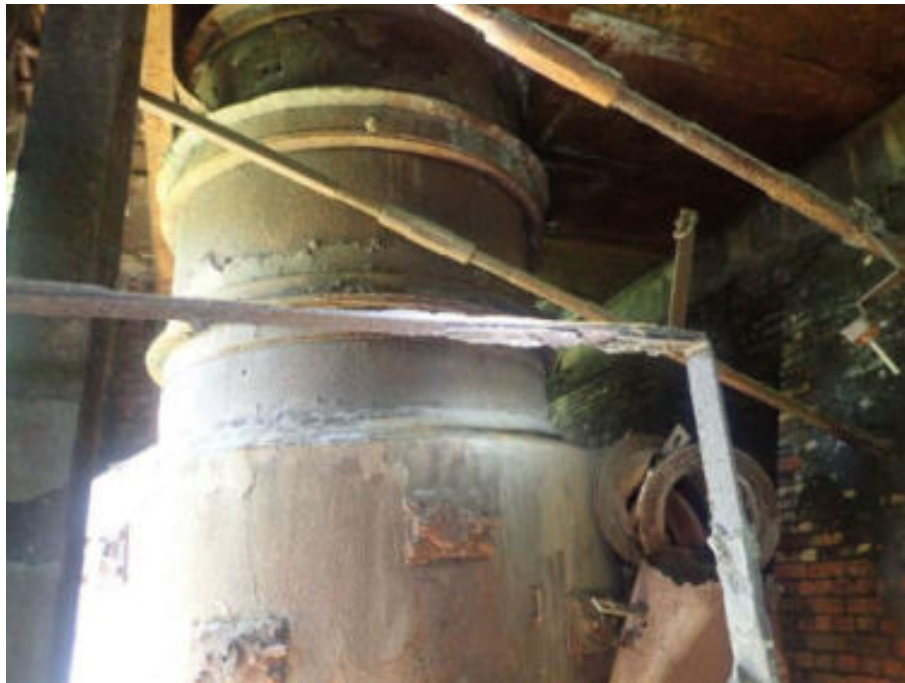
Figure 189. Typical delamination to cupola bases
