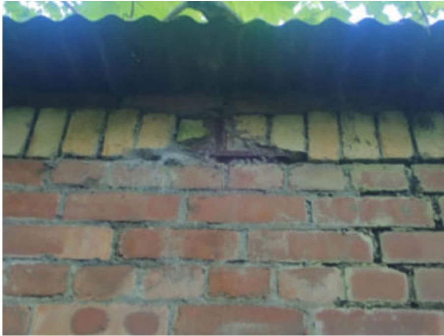
Figure 5. Typical corroded steel truss end
