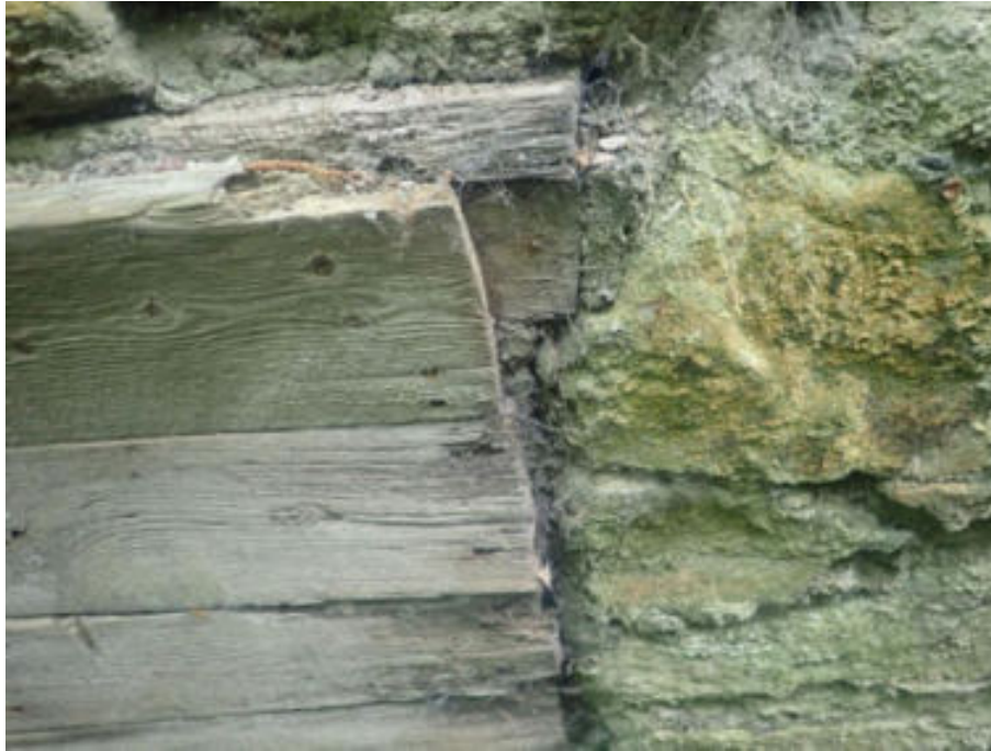
Figure 36. Inadequate lintel bearing
