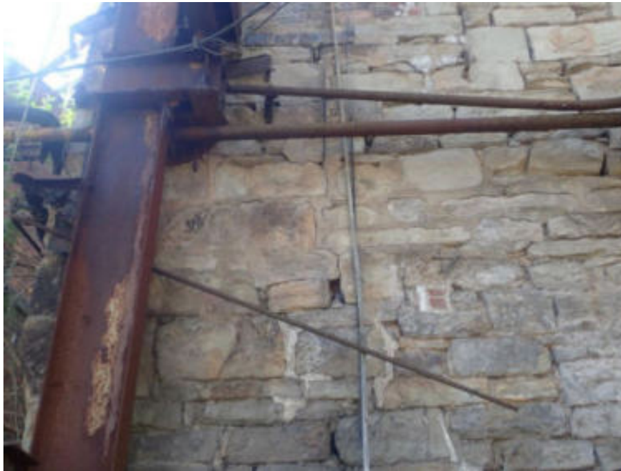
Figure 62. Typical mortar loss
