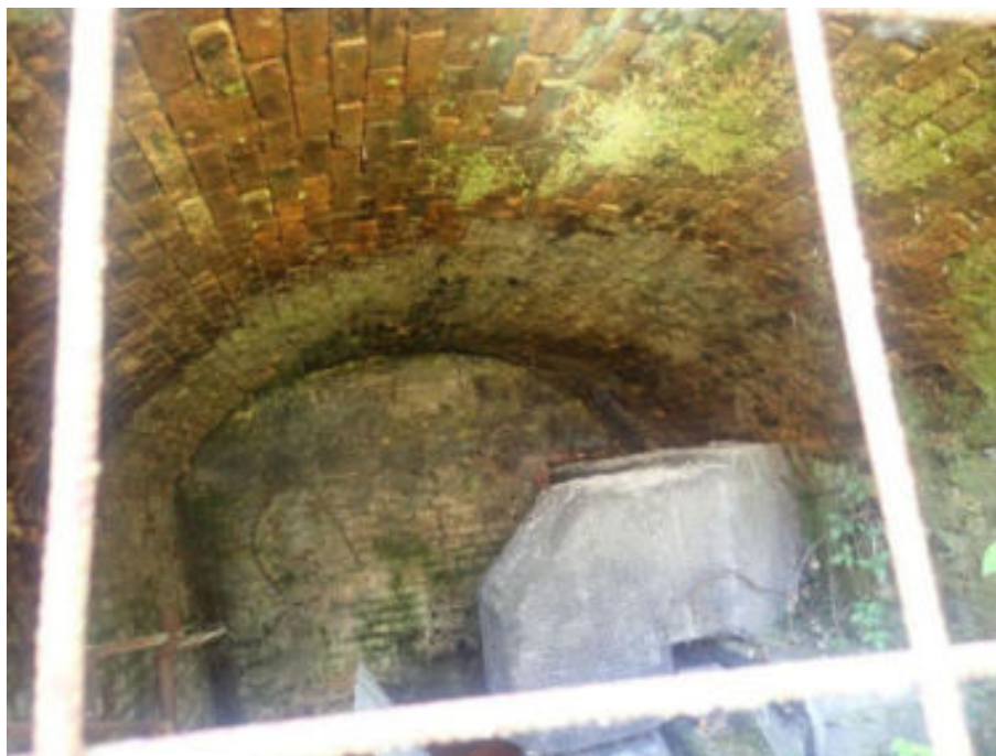
Figure 200. Typical mortar loss
