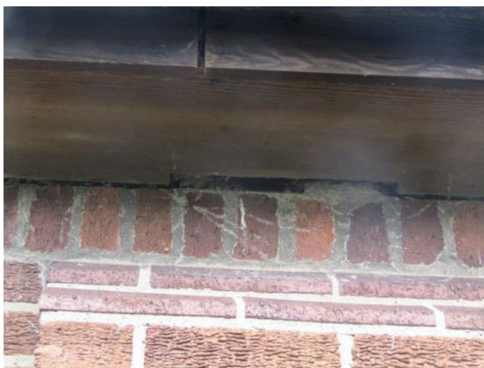
Photo 5: Gap between brick wall and eaves on South elevation.
