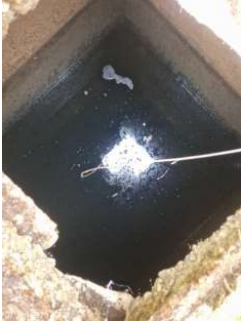
Final Effluent Tank Before Emptying.
