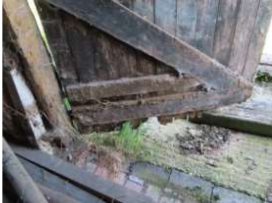
Rot to frame and base of door
