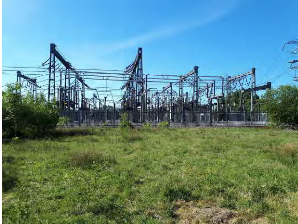
Southern view across the main site with National Grid substation present in the background
