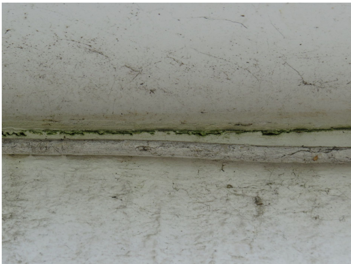
7 – There are no gaps between boxed soffits and render at the eaves.
