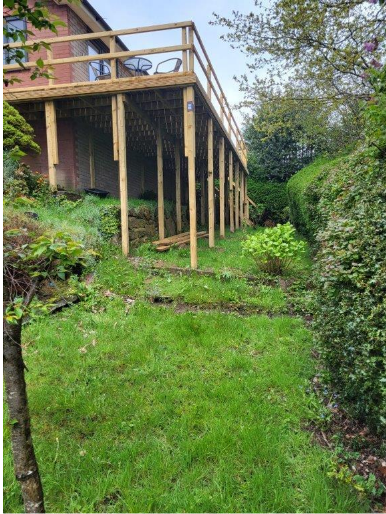
Image 2 – lower garden level, image illustrates the significant drop and previous safety issues
