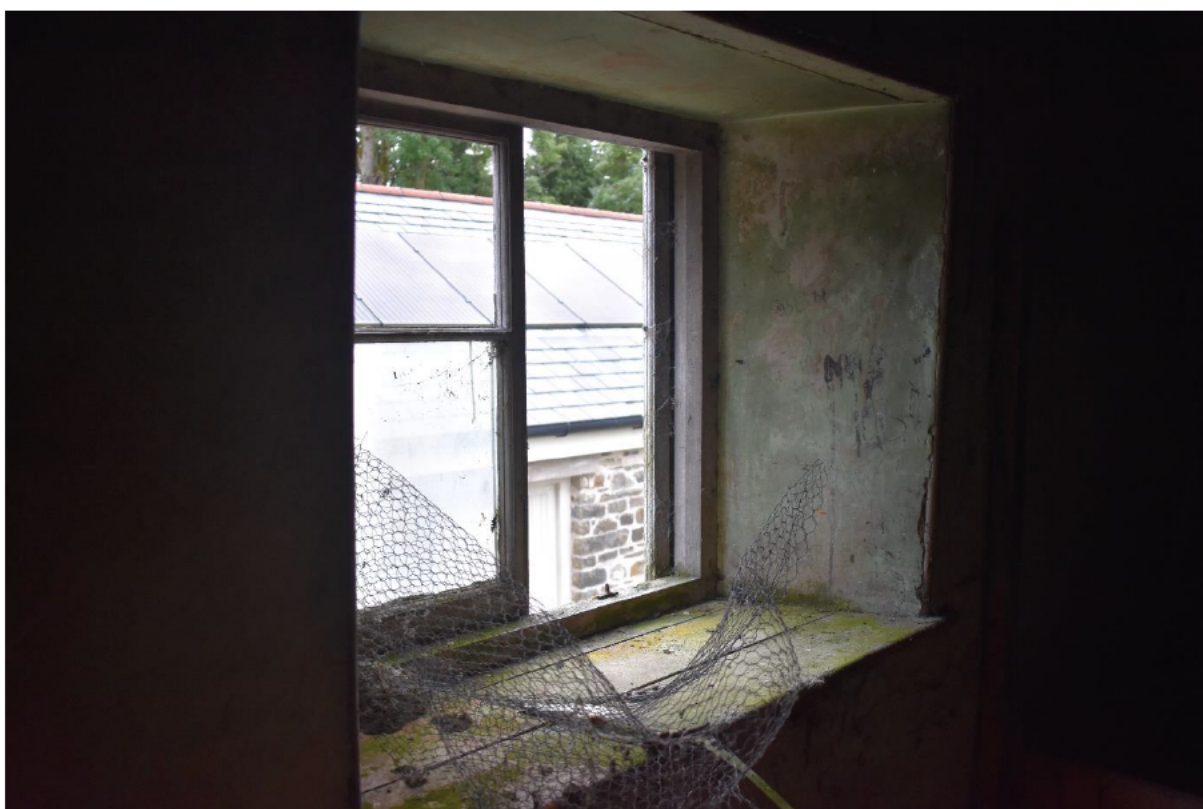
Figure 3.13: The broken window to the above room (within the east-facing gable).
