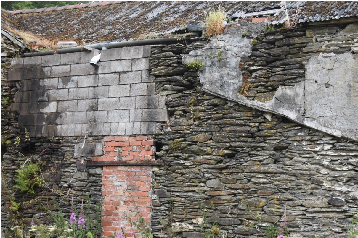
Figure 3.4: The condition of the rear walls.
