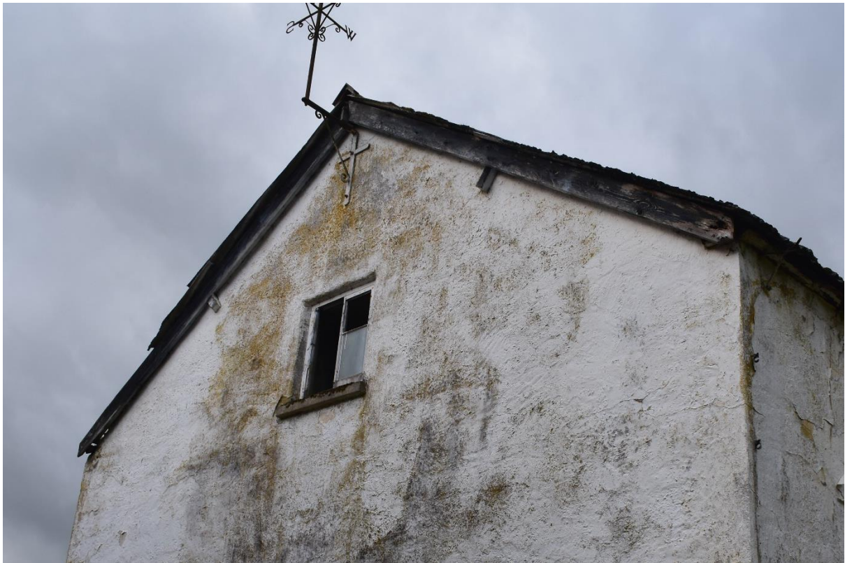
Figure 3.7: The broken first floor window and roofline of the east-facing gable.
