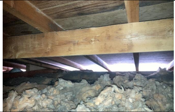
Plate 8: view from the loft looking out of the gaps between the rafters. Note significant light spillage into loft
