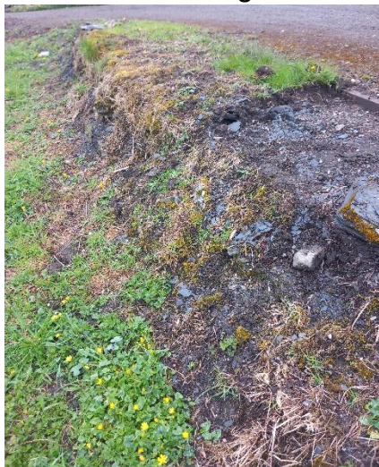
8. Crumbled external garden wall
