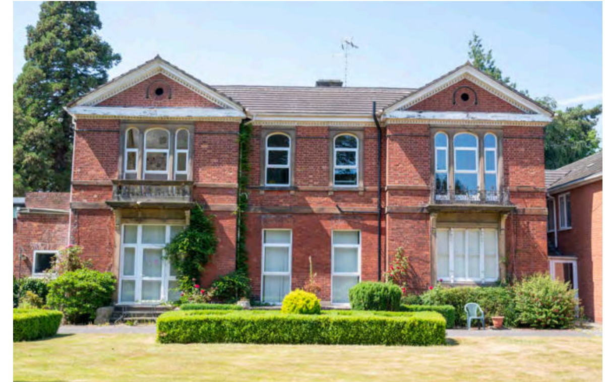
The stone balconies are to be removed as they are currently unsafe and at risk of falling
