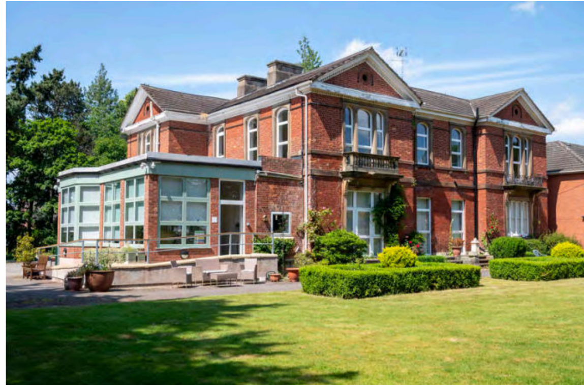
The property benefits from a many historic architectural features, sadly some of these are not in the best state of repair and require attention
