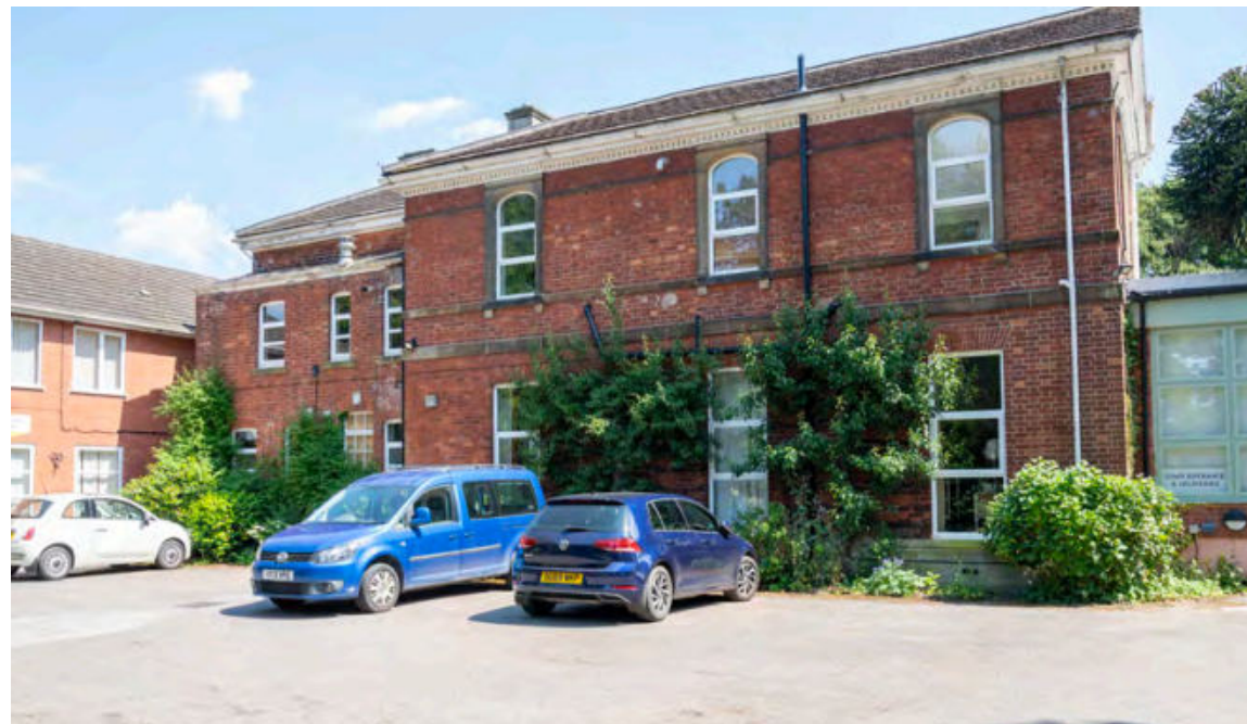
A lack of repairs to the roof has allowed water ingress to parts of the existing brick wall, causing decay. We plan to overclad small section of the Hall to tie in with the proposed extensions
