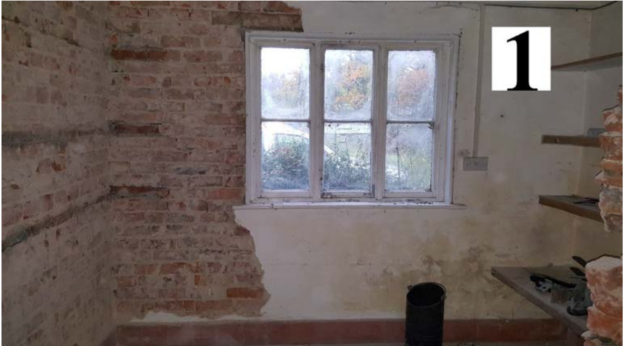
Figure 17 – Further contextual view of pantry shelves which have been lost as part of works already carried out. Photo taken from photographic survey discharged under P/2019/0904.
