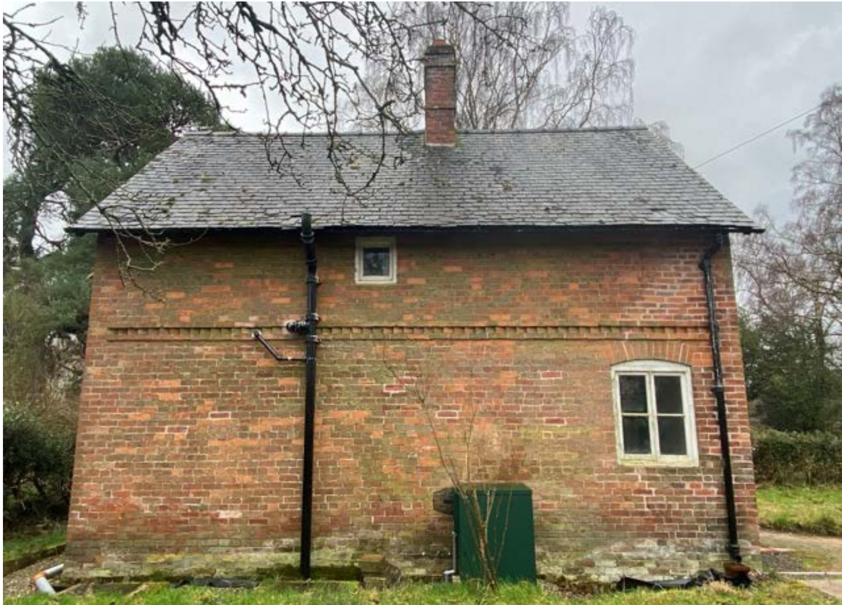
Figure 8 – The northeast elevation of the Site. This Site features the architecturally interesting small, square window, as well as a portion of the dog toothed corbelling detail. However, the presence of the oil boiler detracts from the Site's significance.
