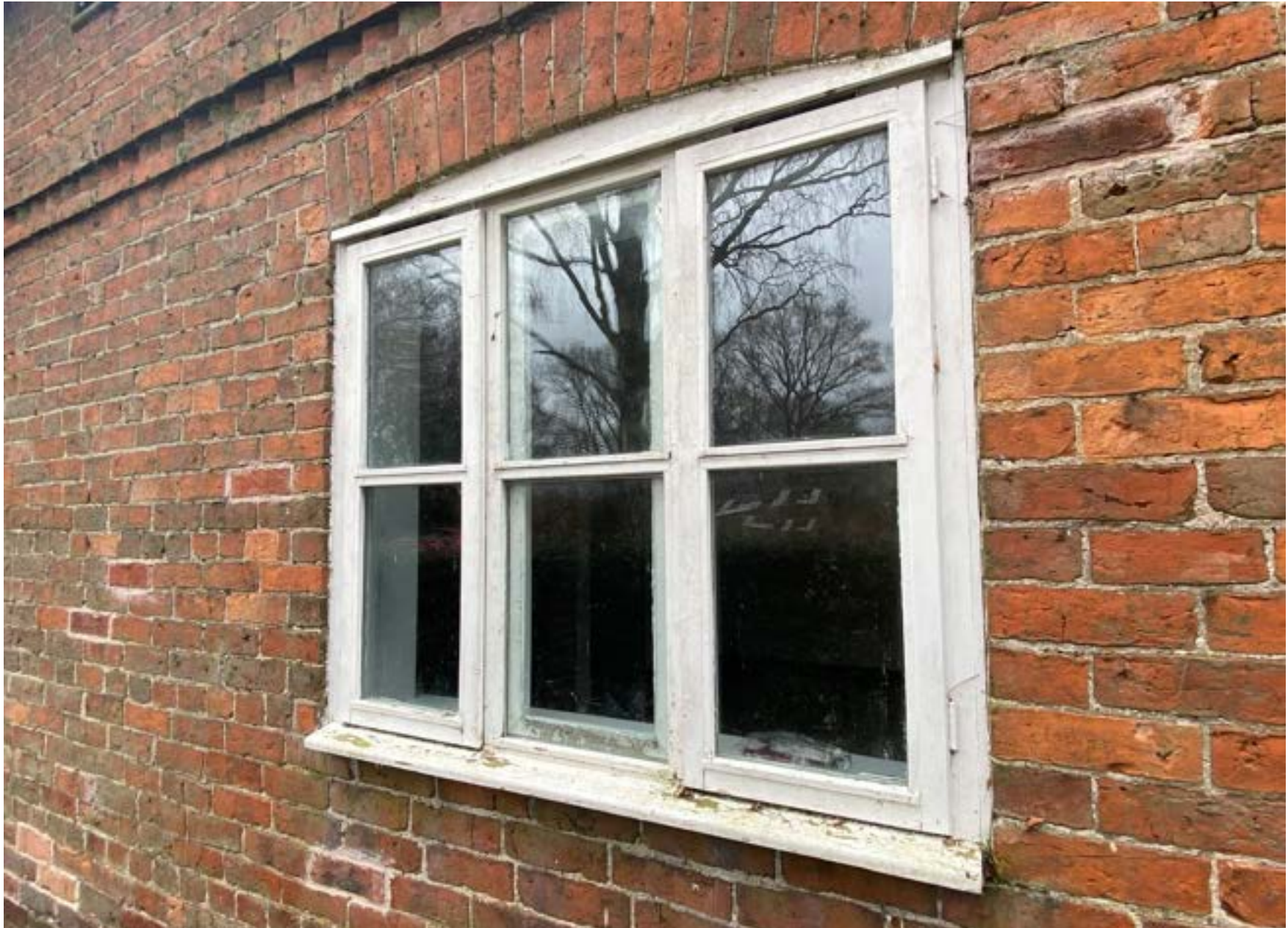
Figure 10 – Window on the southwest elevation has been replaced with a model that is divergent in design from the rest of the Site.
