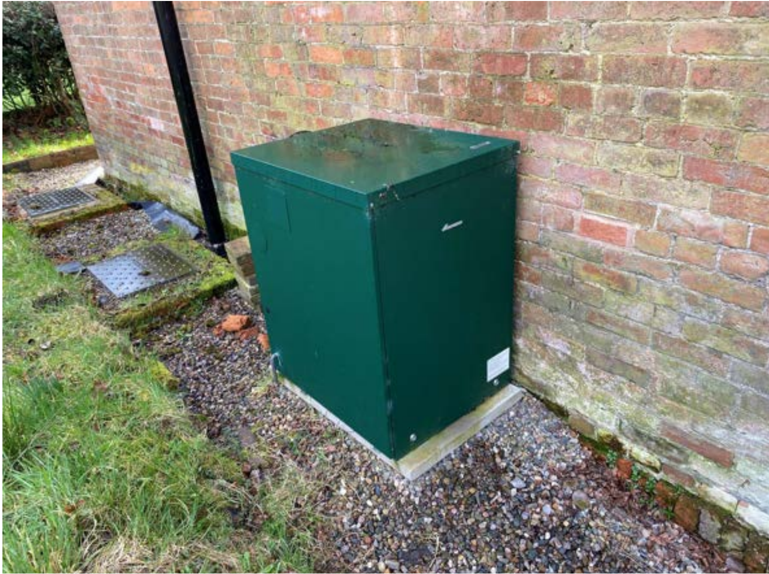
Figure 23 - Unsympathetic oil boiler proposed for removal.
