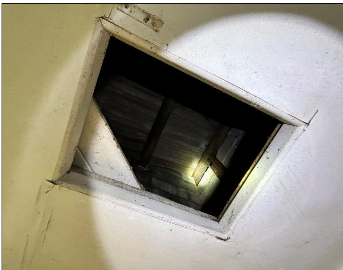
Plate 16 – Void present within south of B2
