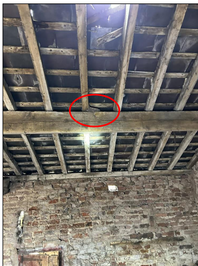
Plate 8 – Gap in the roof of B1, with swallow cup visible
