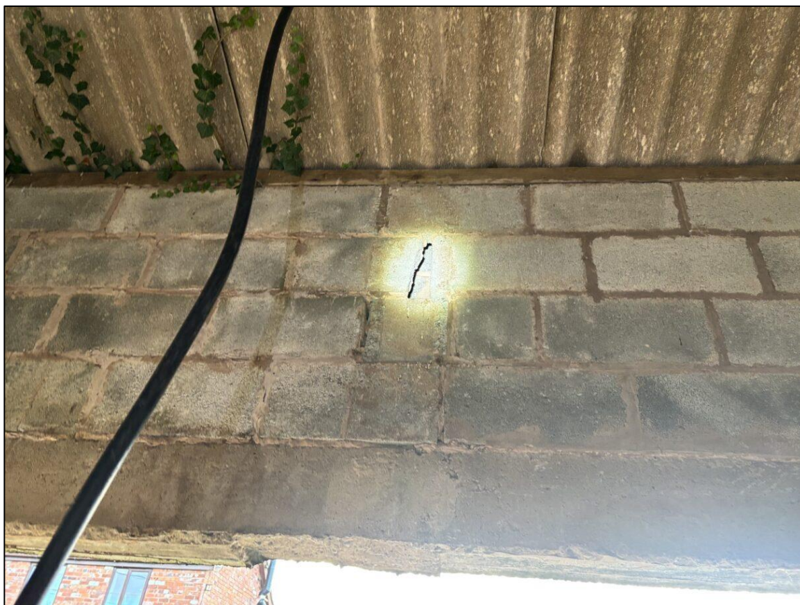
Plate 19 – Viable PRF within B2, leading to cavity wall
