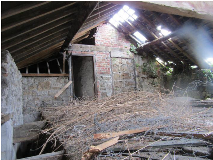
Photo 4: Roof partially collapsed and upper level hay loft floor is rotten.
