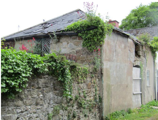
Photo 3: Roof over stable block has holes in.
