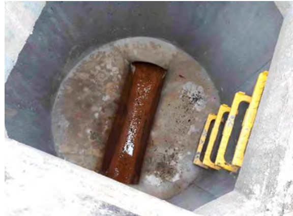
Slight ochreous flow in Foundry Adit drain
