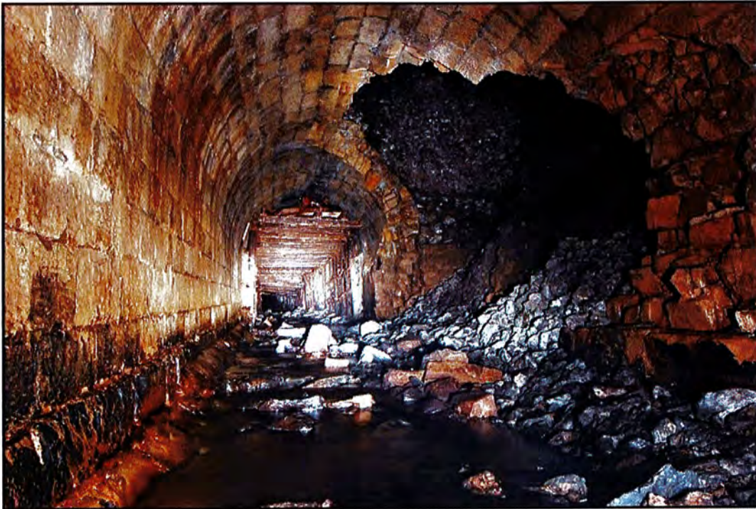
Well-constructed roadway with collapse
