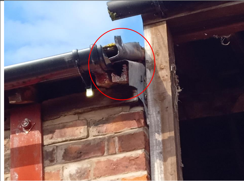
B1 – southern elevation – rot in wood
