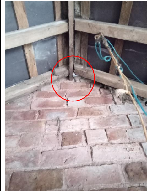
B1 – interior – roof void – gap in tiles
