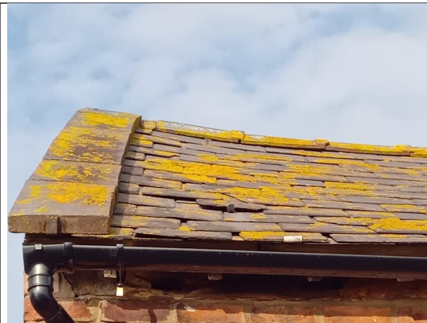
B1 – southern elevation – slipped tiles
