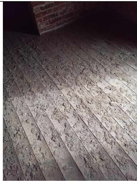
B1 – interior – roof void – bird droppings
