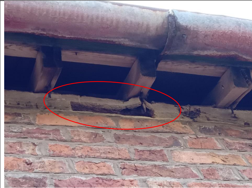
B1 – northern elevation – gap in wood panelling
