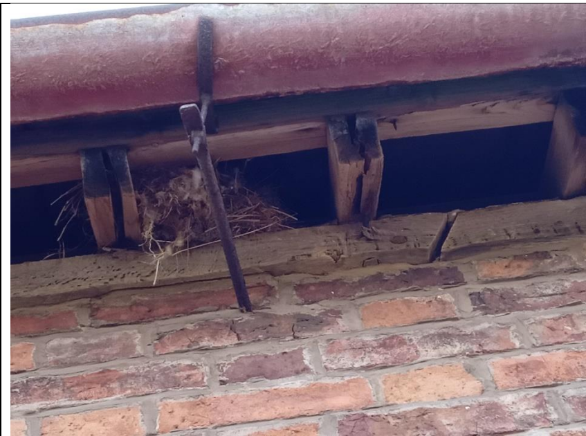
B1 – exterior – northern elevation – birds’ nest in the eaves (potentially active)
