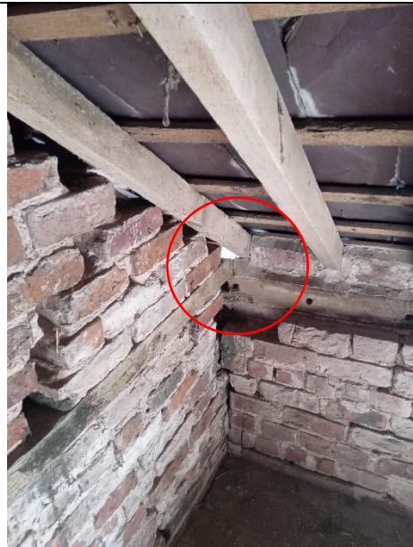
B1 – interior – roof void – gap in tiles
