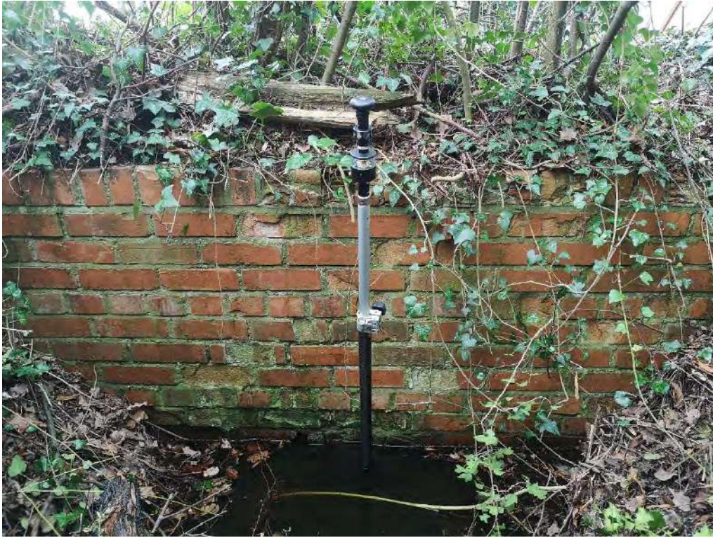
Photograph of the downstream face of blocked Culvert structure Culv_1.19 (NGR 346245 335165):
