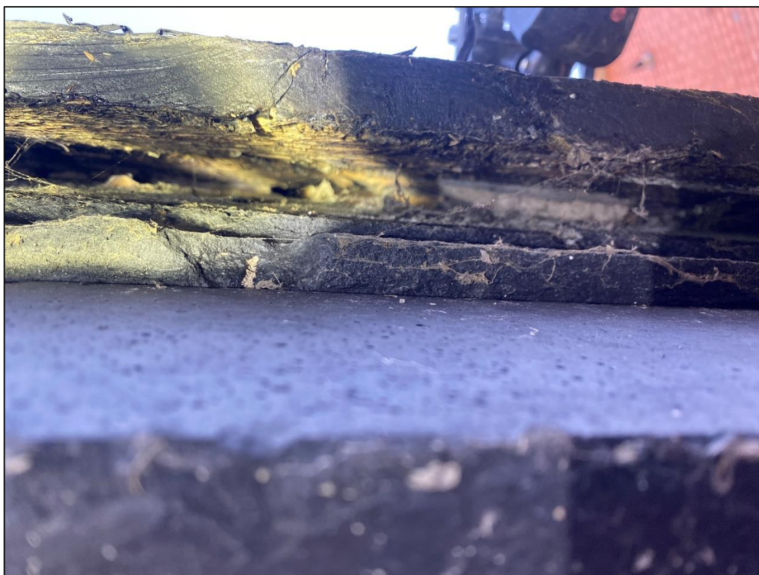
Plate 4 – Nature of crevice beneath fascia of B1
