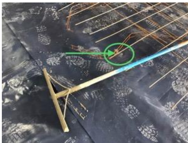
Tool thrown and damaged membrane
