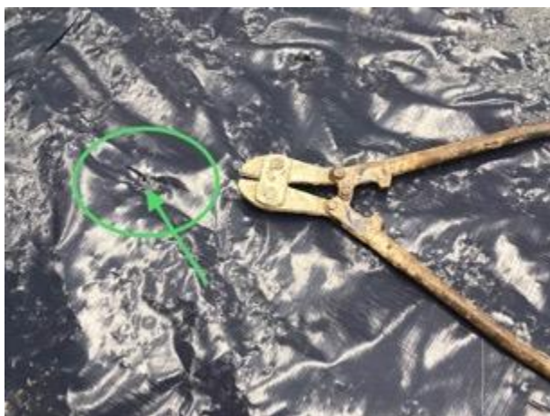
Tool dropped and damaged membrane
