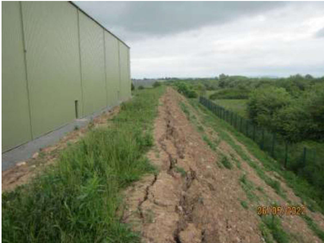
Photo 3. Looking eastwards on inert spoil mound in Extension 1 with large fissures and cracks visible.
