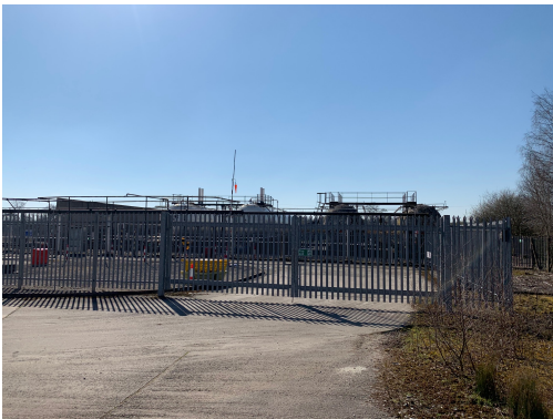
LPG tanks - Exterior Image
