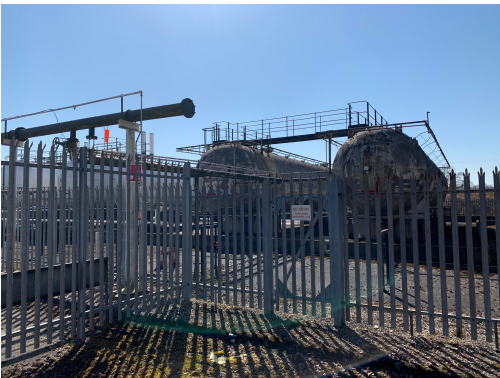
LPG tanks - Exterior Image
