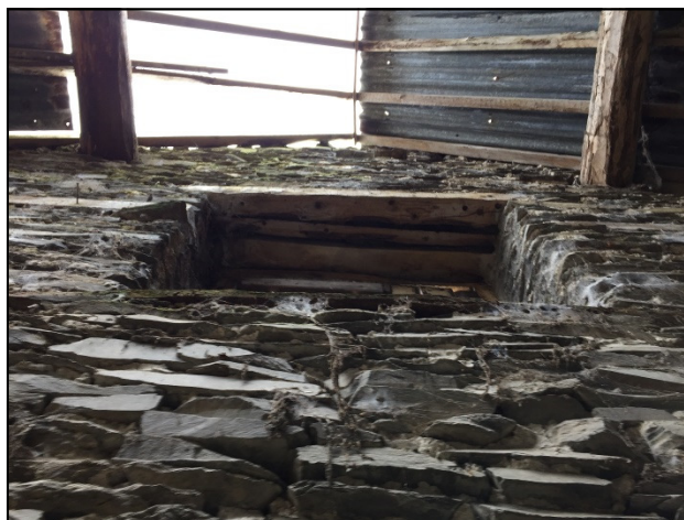
Plate 3 Gaps within timber lintel
