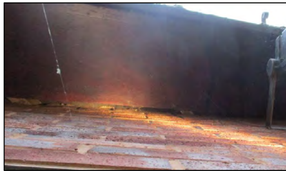
Figure 11: Soffit feature from which bat emerged
