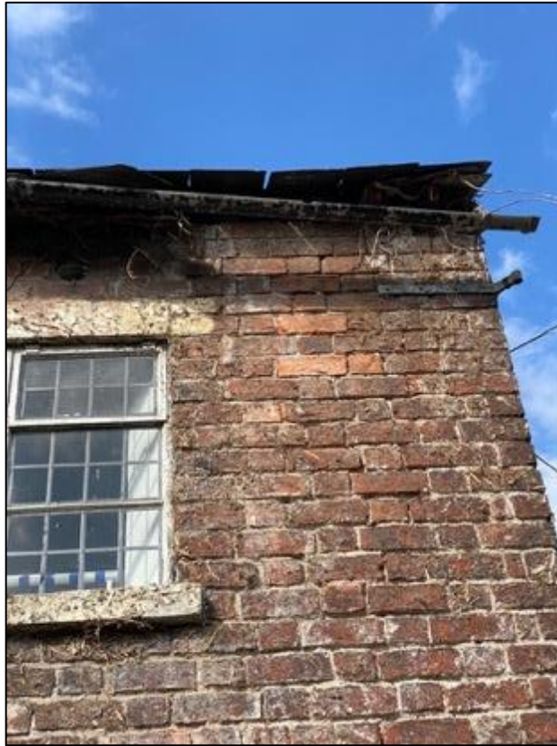
Fig 6: Showing roof damage and more potential entry points for bats into the main target building.
