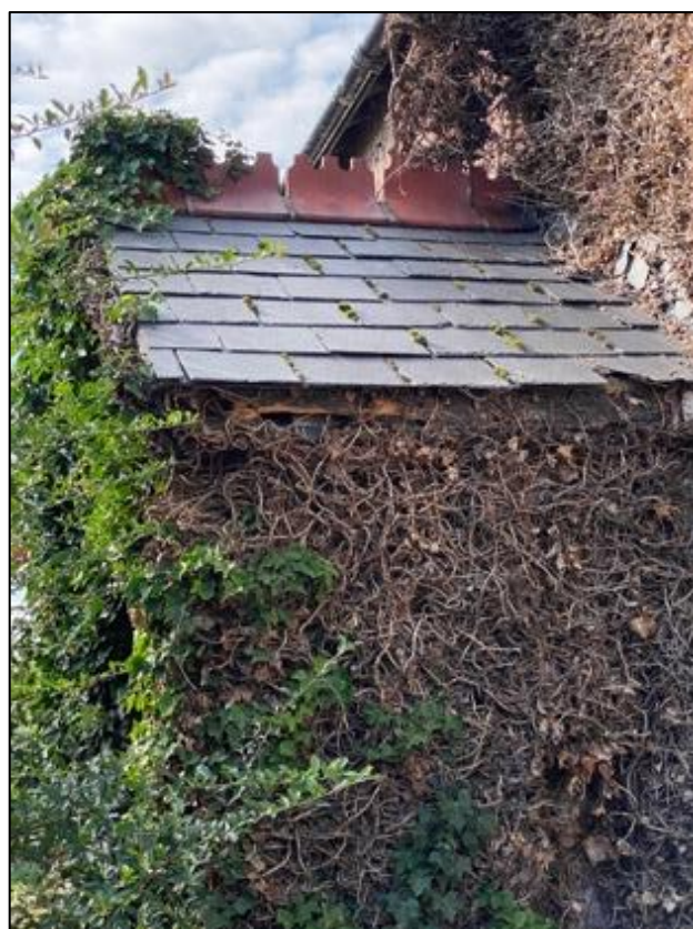
Fig 5: Showing the extent of Ivy encroachment into the front porch of the property leading directly inside.
