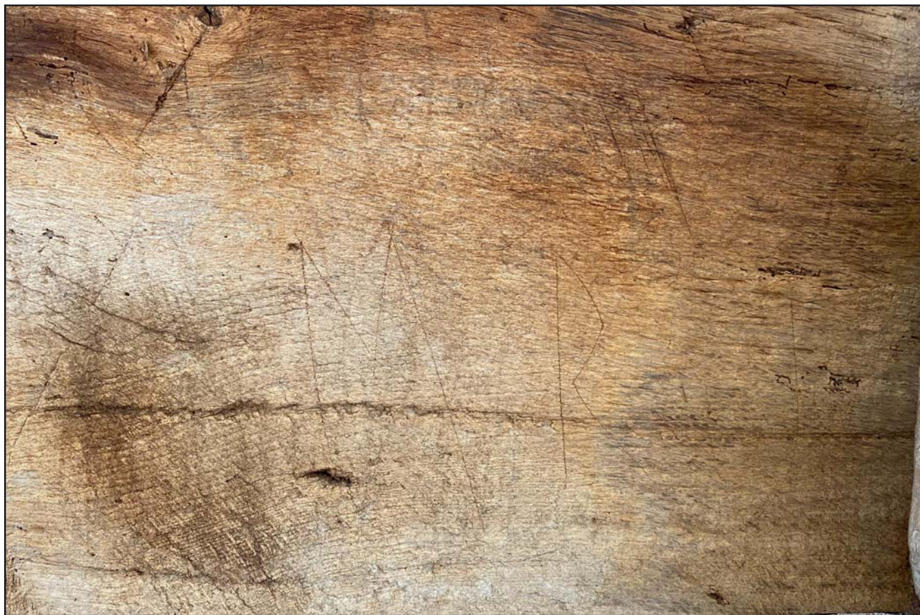
Plate 72: Faint Apotropaic Marks on northwest side of handhewn tie beam: Marian & Hexafoil? Truss 2, within Shippon 1 at Brunette Farm, Ty Broughton, Wrexham - from the southwest - no scale
