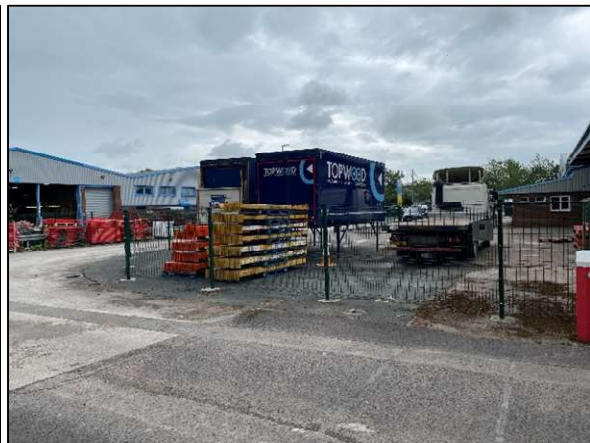
Figure 9: Further stored materials on site.
