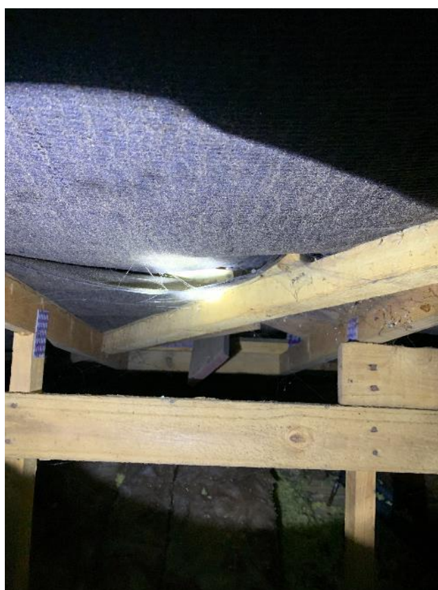
Plate 10 – Evidence of deterioration in bitumen 1F underfelt
