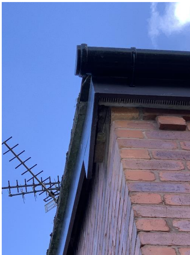
Plate 7 – Gap behind barge boards on the northern elevation
