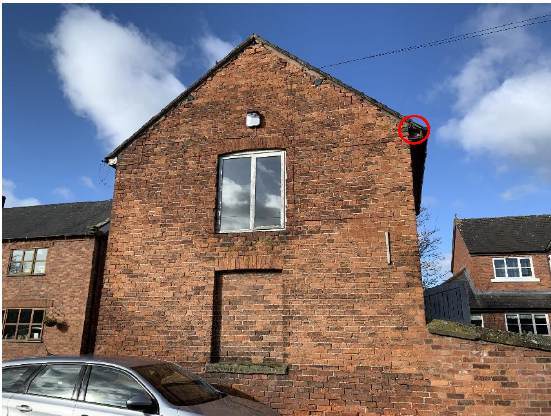
Plate 15 – Eastern elevation of B2, with gap behind soffit circled
