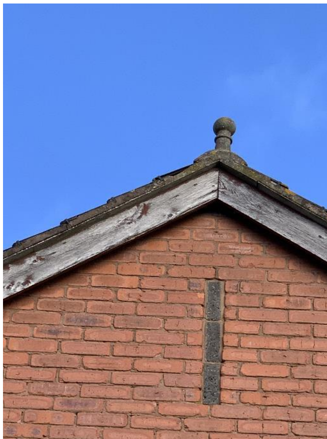
Plate 3 – A gap below the roof tile on the southern elevation
