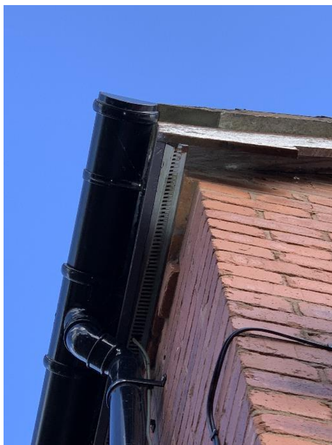
Plate 4 – Gap behind the soffit meshing on the southern-western interface
