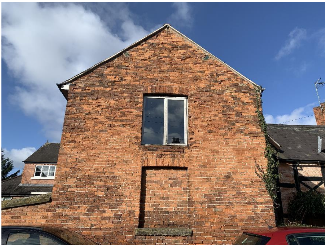
Plate 21 – Eastern elevation of B3, with entry points in the brickwork, along the gable and surrounding the timbers
