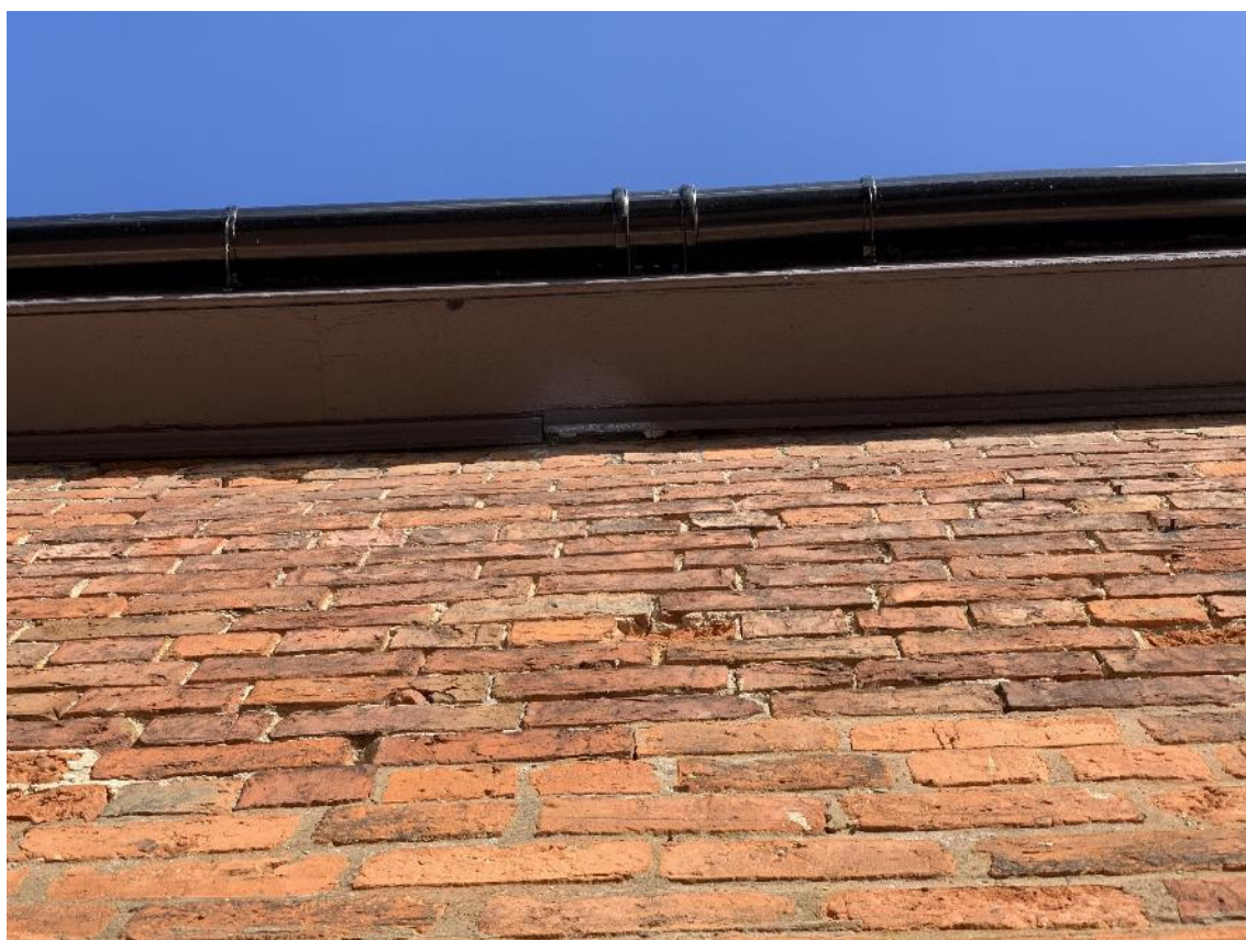
Plate 20 – Gap behind soffit box on southern elevation
