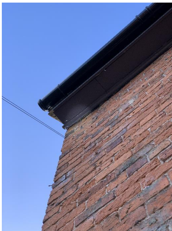
Plate 12 – Gap behind soffit on the northern elevation
