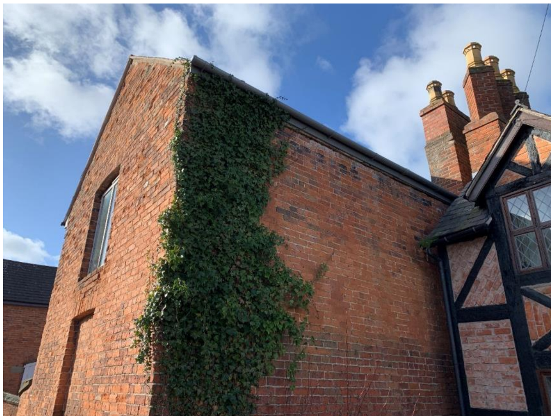
Plate 23 – Northern elevation of B3 with ivy present and gaps behind timber fascia
