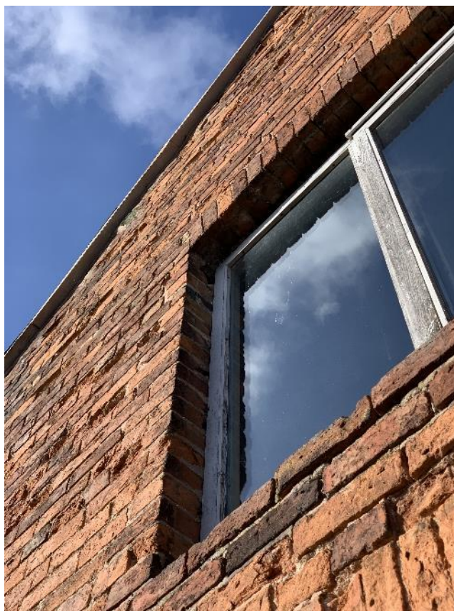
Plate 22 – Gap above window in the brick lintel
