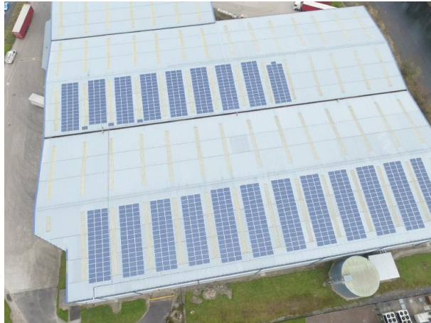
Figure 3: Typical roof mounted PV panels on a warehouse roof
