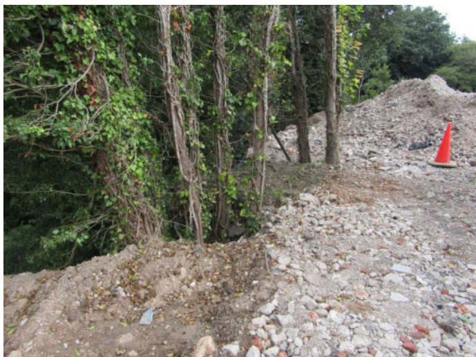
Photo 4: Sycamore and Alder trees with rubble piled around trunks.
