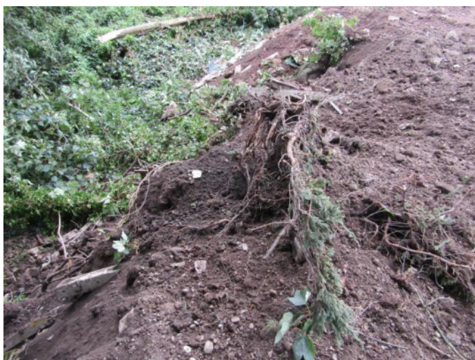
Photo 6: Soil and rubble on edge of infill.
